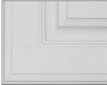
Example of front joint separation
