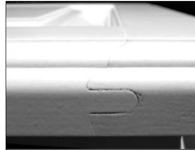
Example of end joint separation
