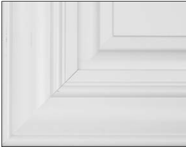
Example of front joint separation
