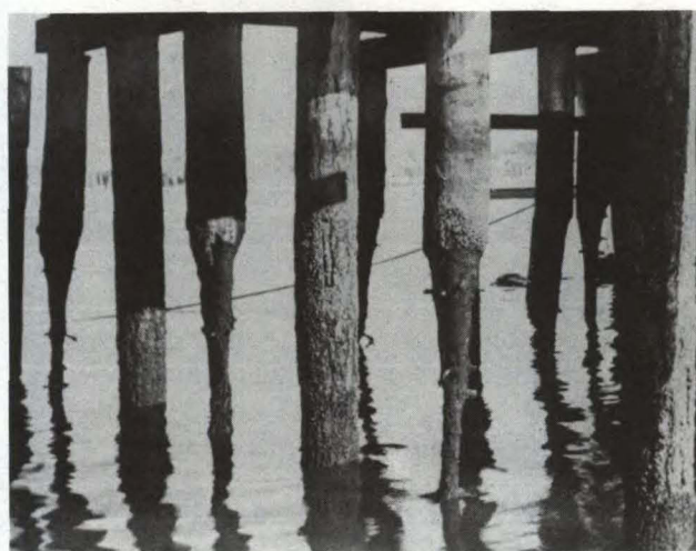
FIG. 46. Pencil pointed piling resulting from gribble attack along with replacement piles. (From Hill and Kofoed 1927)
