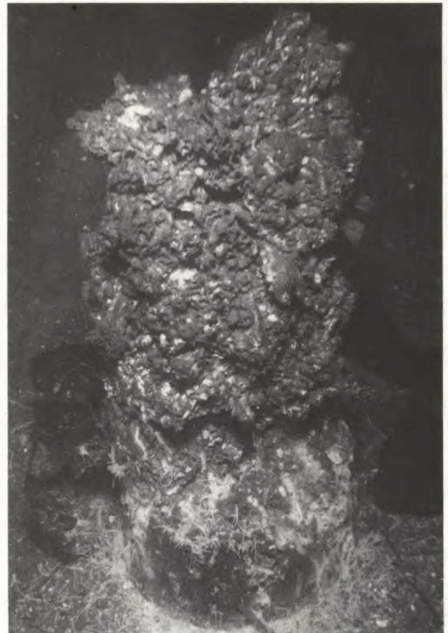
FIG. 38. Remains of an untreated fir control pile destroyed in less than 2 years in the 1969 Crofton piling protection study. Note frass at the base of the pile. (Underwater photograph. P. Fraser)
