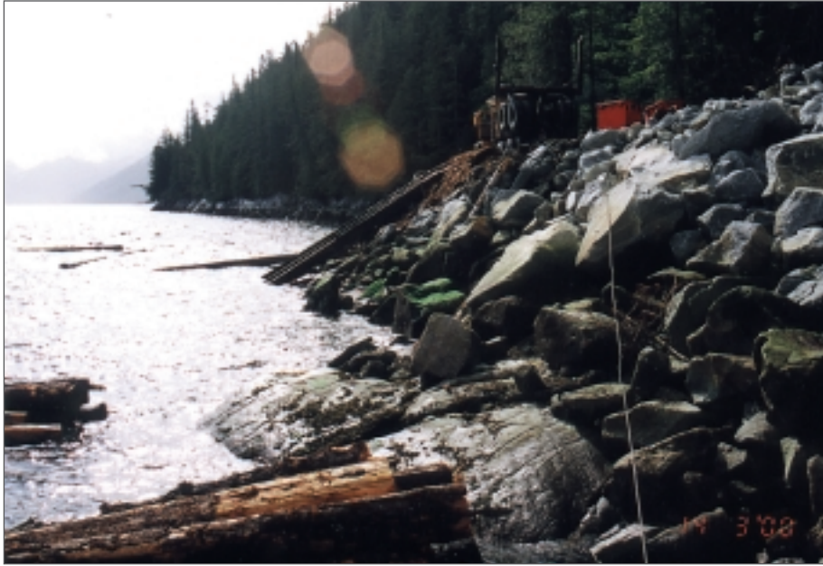
Photo 16: East Gribbell Island log dump, fill upslope of bedrock along foreshore; logs in contact with shoreline (March 2000).
