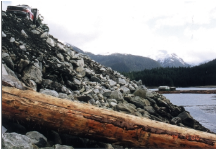
Photo 22: Goat Harbour log dump, fill used in construction of the dump ramp (March 2000).
