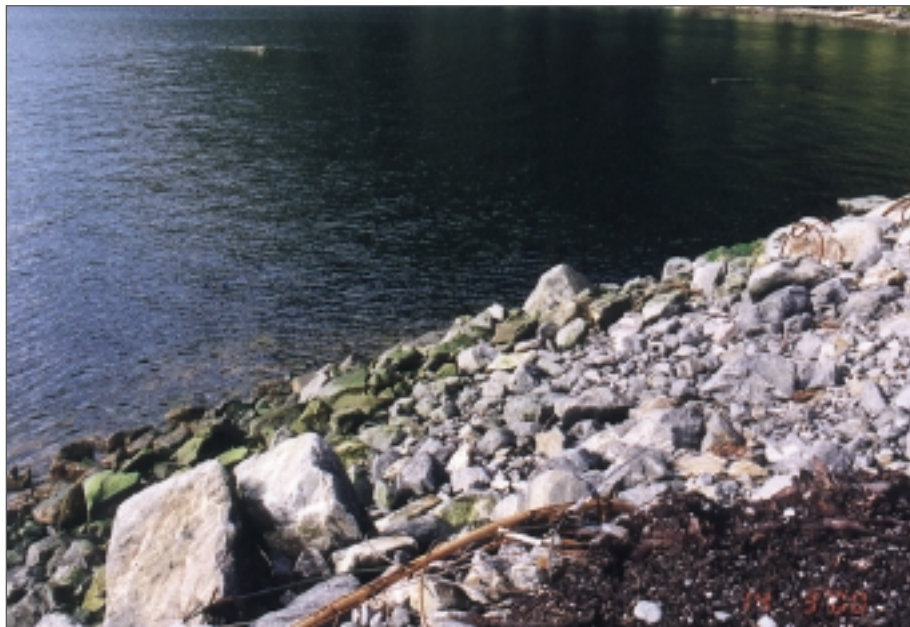
Photo 42: Verney Pass Creek dumpsite, smaller-sized fill used to extend barge ramp (March 2000).
