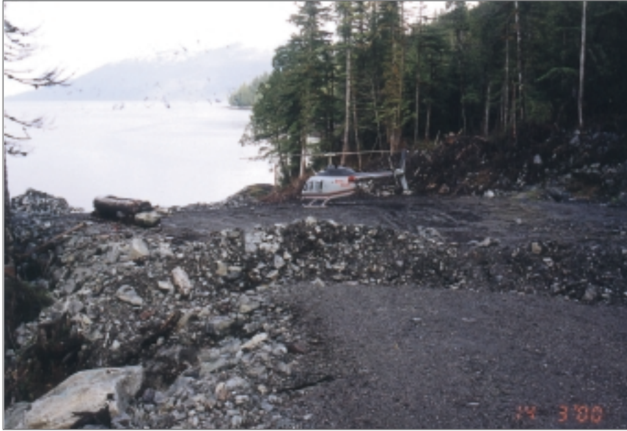
Photo 33: Cross bar installed during partial deactivation of Verney Passage log dump (March 2000).
