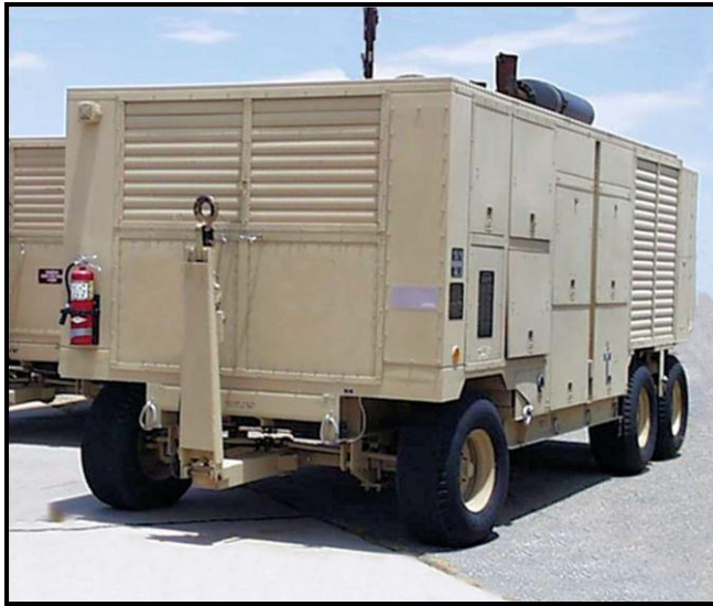
Figure 7.6. MEP-012A 750-kW Generator
