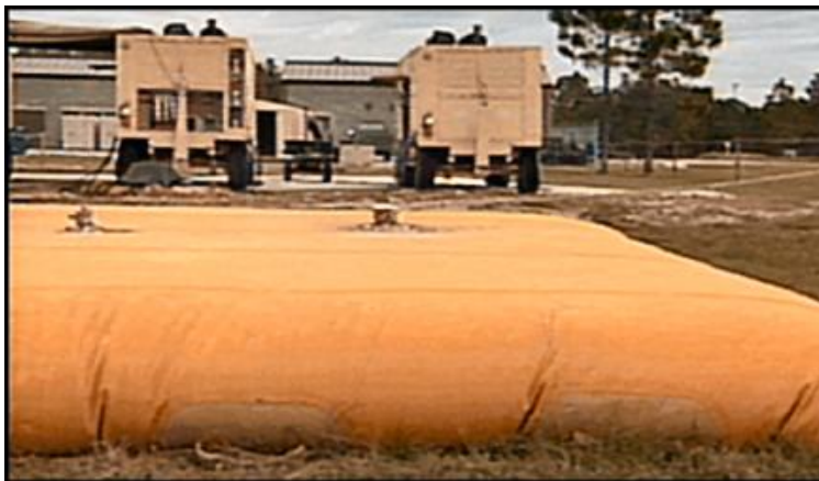
Figure 7.7. Generators with 10,000-Gallon Fuel Storage Bladder
