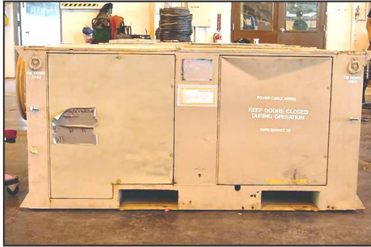
Figure 11.12. A/E32C-39 Environmental Control Unit
