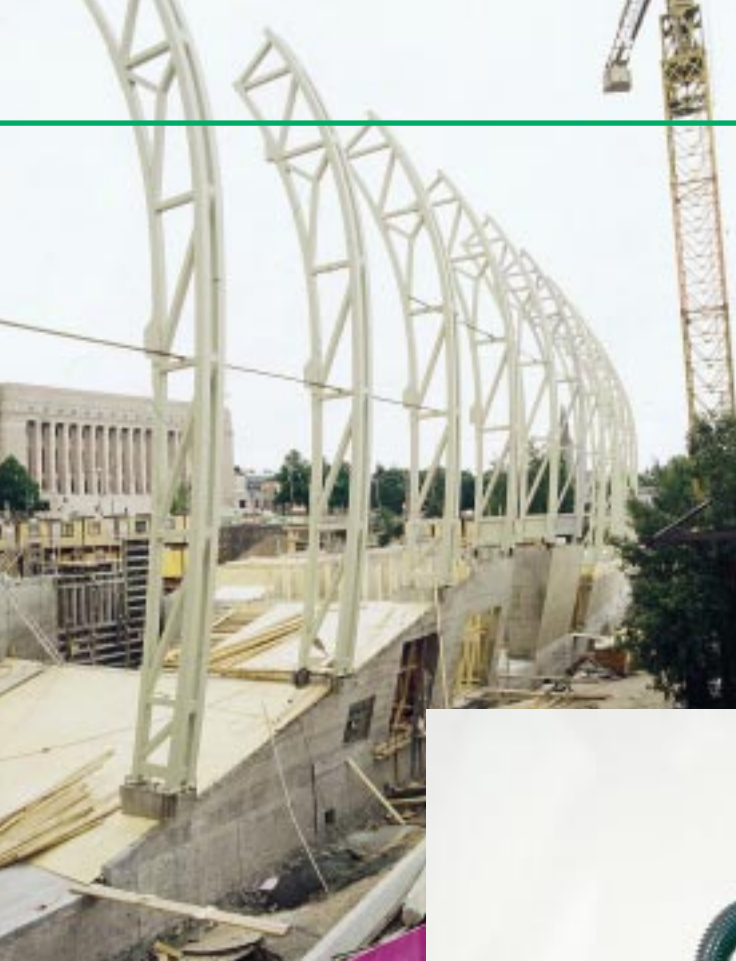
Metform's hollow sections give Helsinki's new Museum of Modern Art its structural rigidity.
