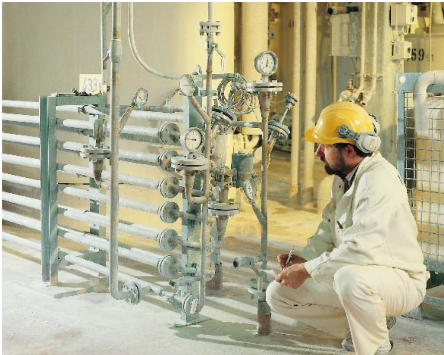
Demand for titanium dioxide was brisk and producers' capacity was in full use. Kemira Pigments is boosting its production capacity through debottlenecking. (Photograph: Seppo Kaksonen)
