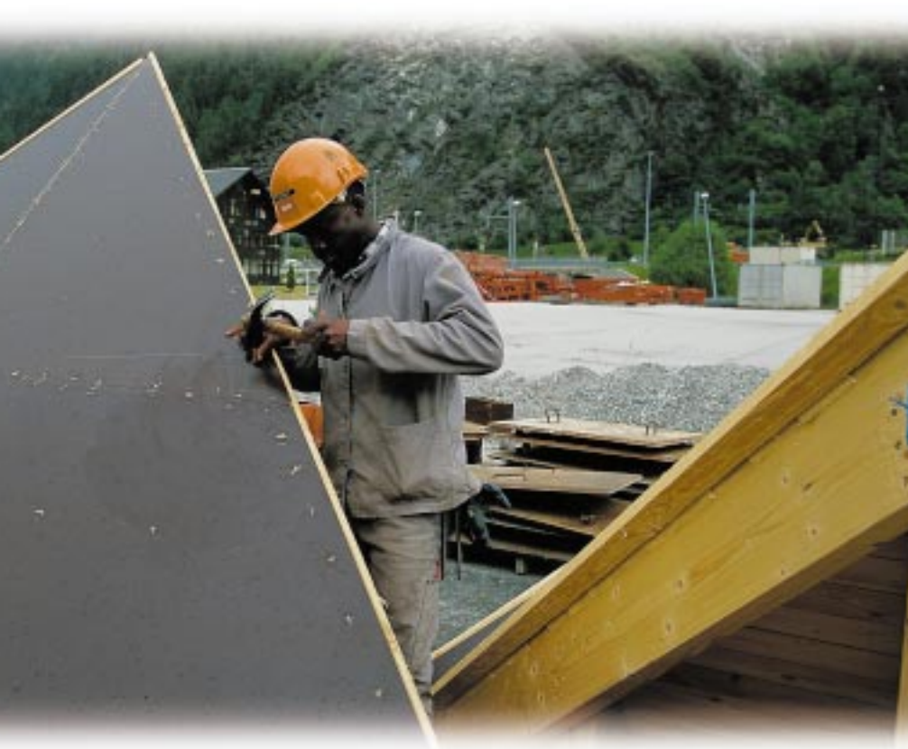
Schauman Wood's Wisa-Form plywood was used as shuttering board on this bridge construction site in France.
