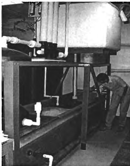
Photo 3. Bead filter, UV sterilizers, head and sump tanks.
