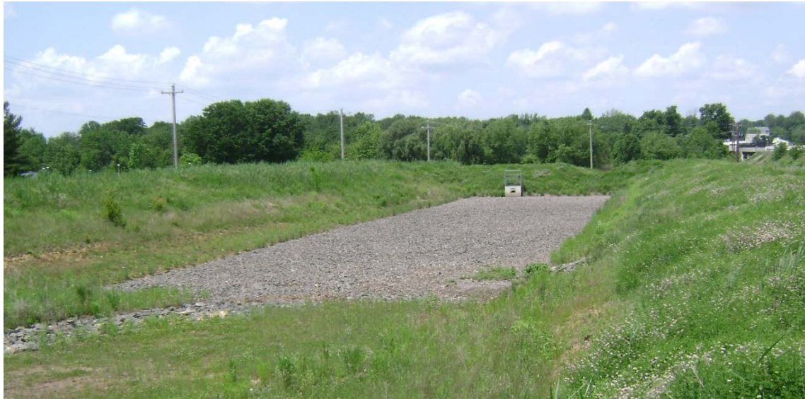
Figure 6.3.1: Infiltration Detention Basin with Engineered Soil Surface (photo c/o: PennDOT)
