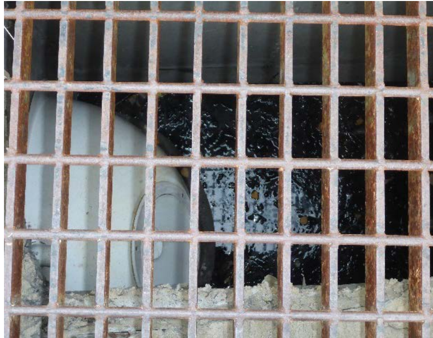
Inlet with Sump/Hood
