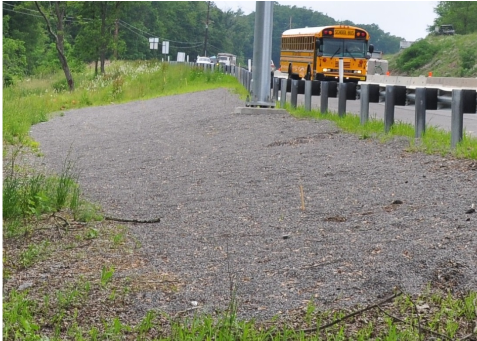
Figure 6.10.1: Media Filter Drain with Unvegetated Surface (photo c/o: PennDOT)
