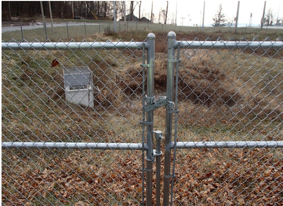
Figure 5.2.1: Fencing Surrounding an SCM (photo c/o: PennDOT)
