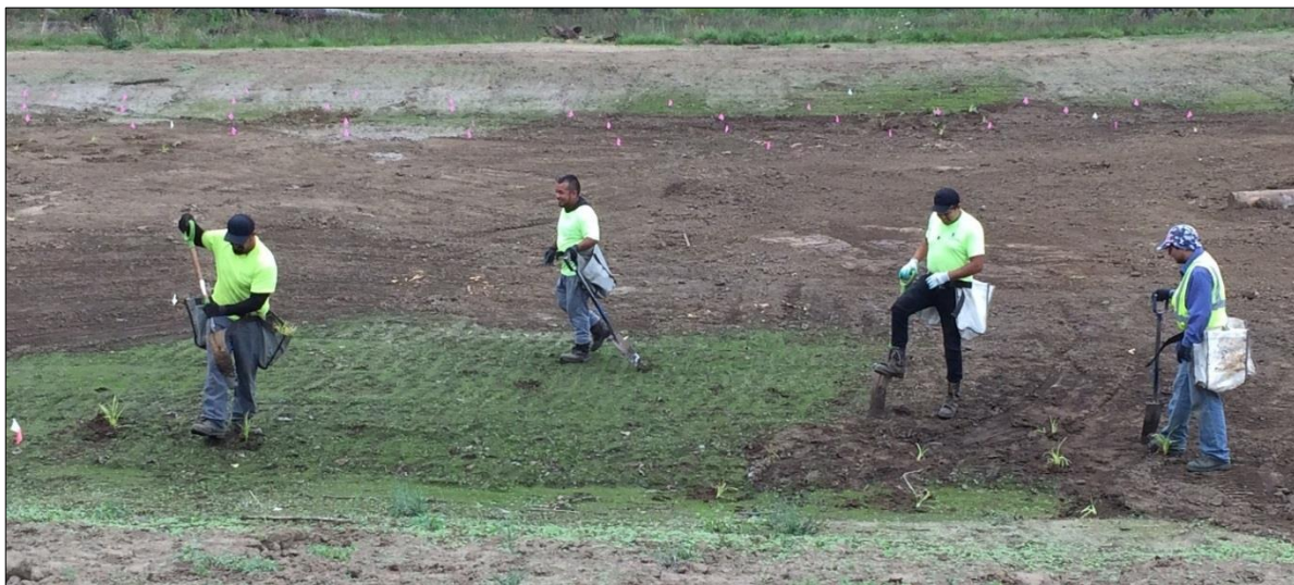
At the Carli Creek enhancement project site, contractors installed emergent wetland plants in a constructed wetland for stormwater treatment.
