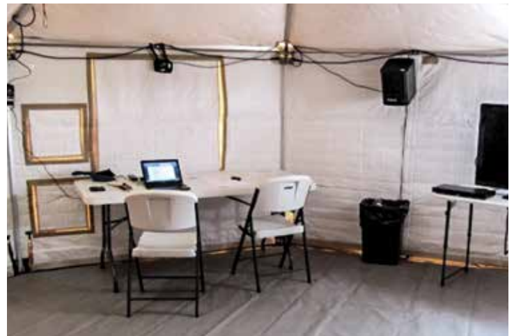
Air Purifier installed in a 1935 Shelter System
