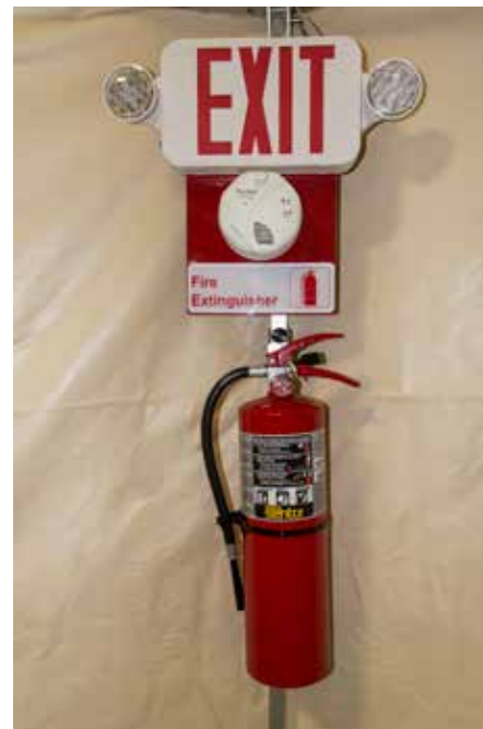
Safety Kit mounted conveniently on wall of shelter.
