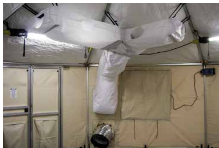
Plenum installed in SH-20 shelter
