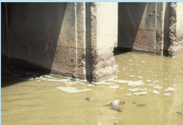
Concrete bridge pylons in the Pimpama River, south-east Queensland, corroded by acid sulfate soils
