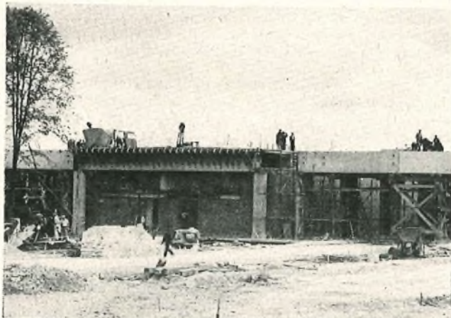
EARLY STAGE OF THE CONSTRUCTION OF THE NEW TERMINAL BUILDING, SHORTLY BEFORE THE INSTALLATION OF POST OFFICE EQUIPMENT
