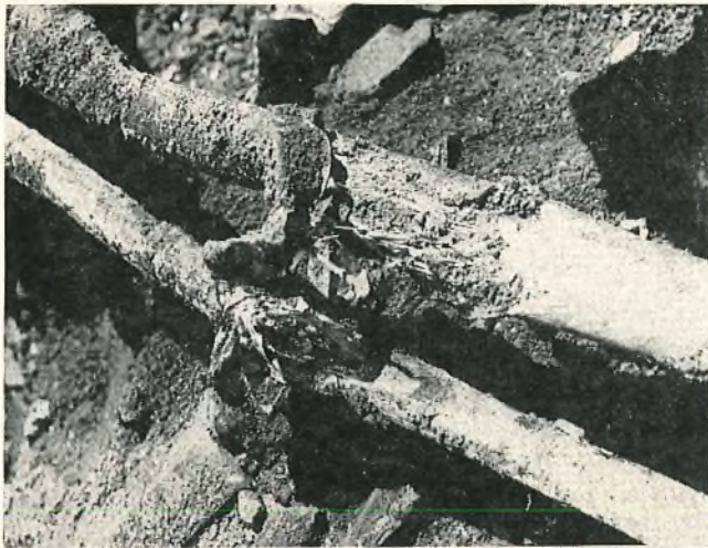
DAMAGE TO CABLES AT TRENT VALE
