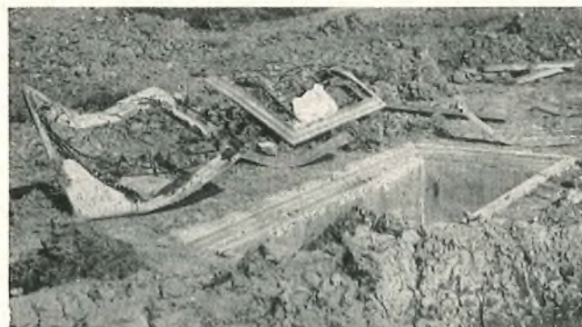
SURFACE JOINT-BOX DAMAGED BY LEVELLING MACHINE
