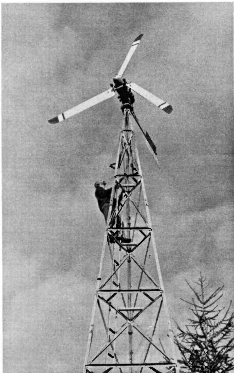
Climbing the tower to check that all is well with the three bladed generator.
