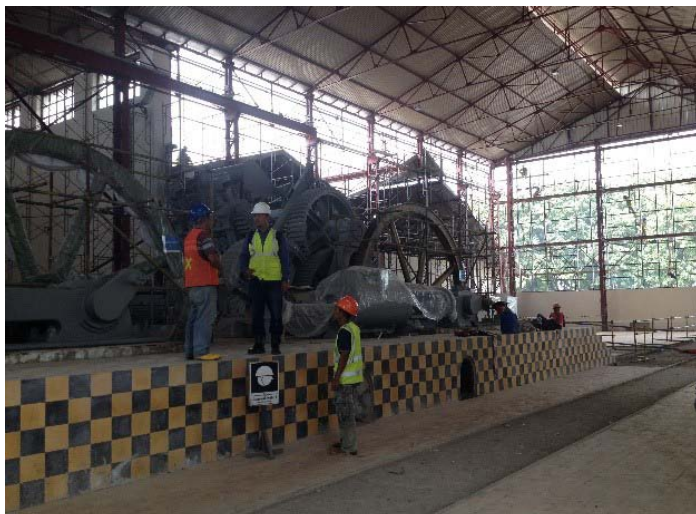
Tjolomadoe Former Sugar Factory during renovation in 2018, Surakarta, Central Java. (Hasti Tarekat)
