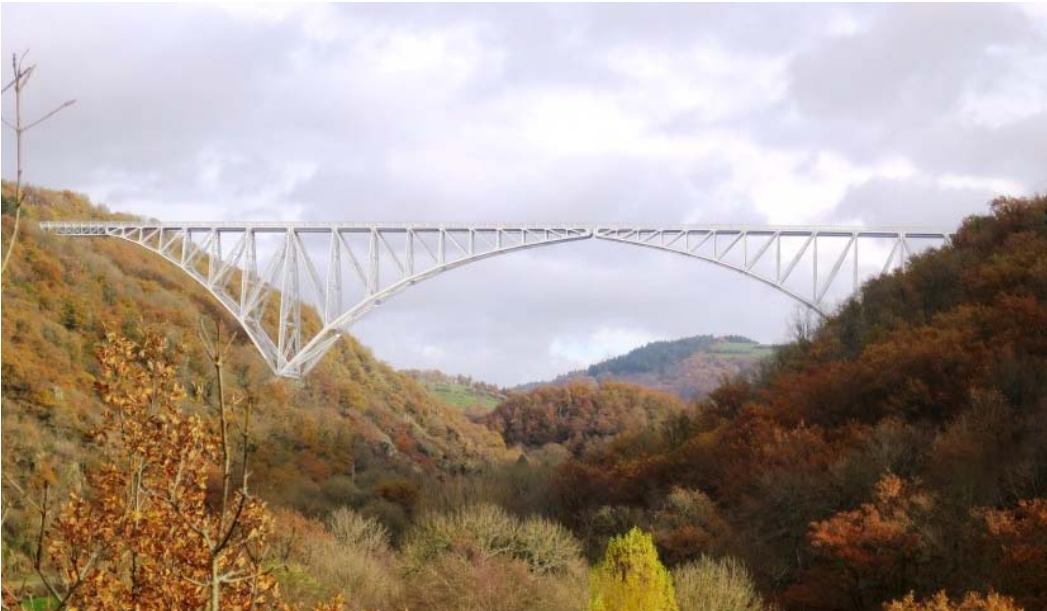
The 1902 Viaur railway viaduct designed by the engineer Paul Bodin, 'classified' as a historic monument in 2021. (Paul Smith)
