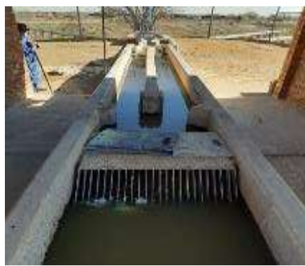
Screening is not optimal and screenings/grit disposed and burnt on-site
