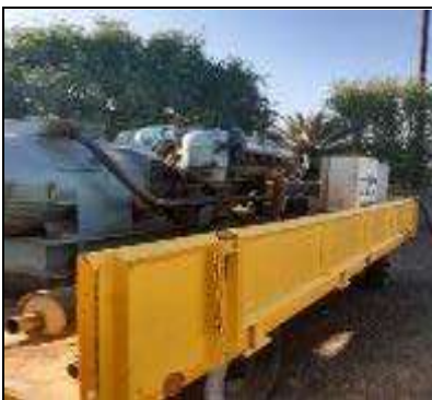
Vacuum tankers discharge wastewater to the head of works
