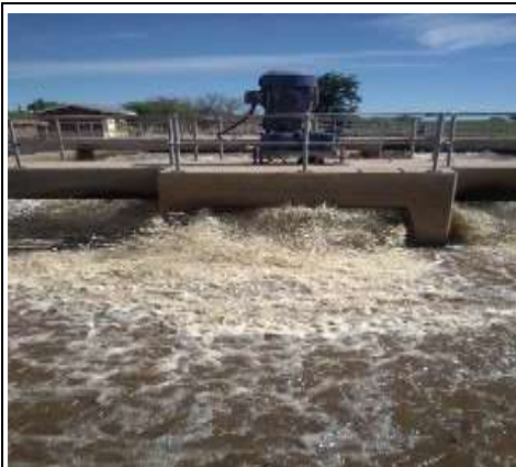
3 of 4 aerators functional at activated sludge plant – operational monitoring done by internal lab
