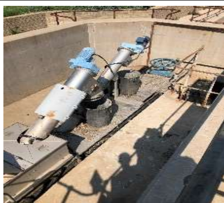
Screening and de-gritting installed at head of works
