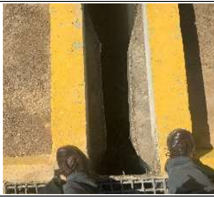
Flow through grit channels controlled by standing way flume. Flume not effectively constructed, rendering it ineffective to control flow
