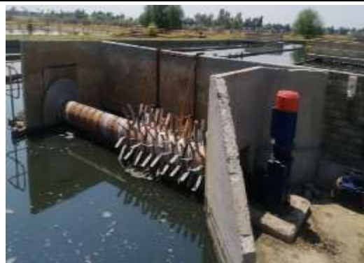
Mechanical equipment not operational due to lack of maintenance and servicing
