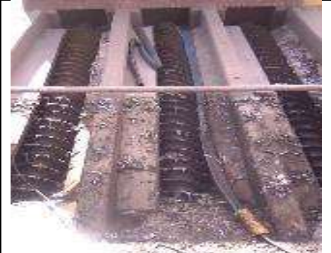
Mechanical screen and RAS archimedes screw pumps are repaired – 2 months lead time
