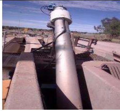
Mechanical screen and RAS archimedes screw pumps are repaired – 2 months lead time
