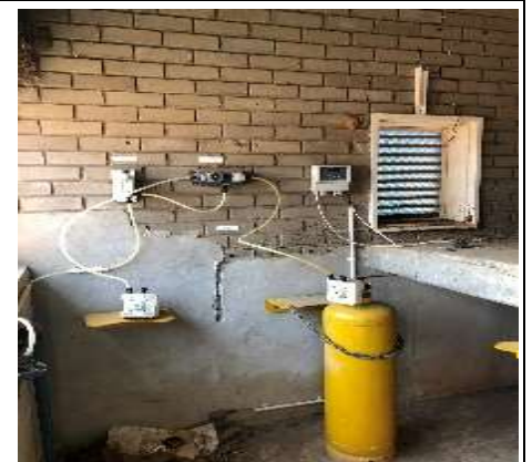
Existing disinfection facility being extended to sodium hypo chloride, will be commissioned under the current upgrade contract
