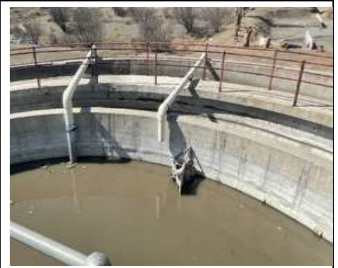
The biological reactor has been non-operational for 4 years
