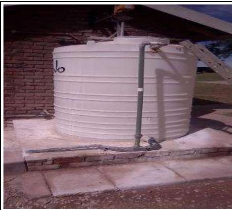
Jo jo tanks used to dose chlorine tablets manually
