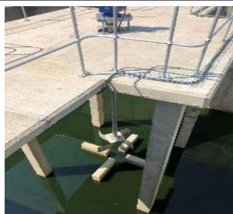
Commissioning of the new unit processes will enhance treatment capability and improved final effluent quality
