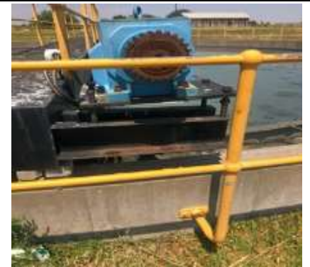
Mechanical equipment not operational due to lack of maintenance and servicing
