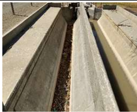
Grit channels not cleaned regularly
