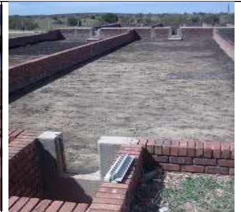
Sludge drying beds in good condition and well operated
