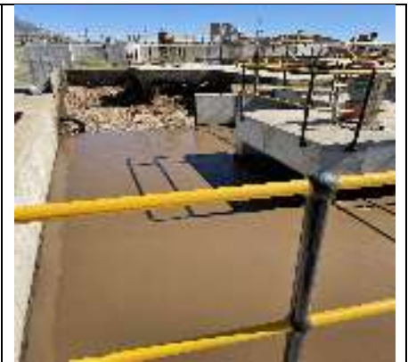
Aeration basin with all aerators in working order – excellent biomass. Highly competent Process Controllers
