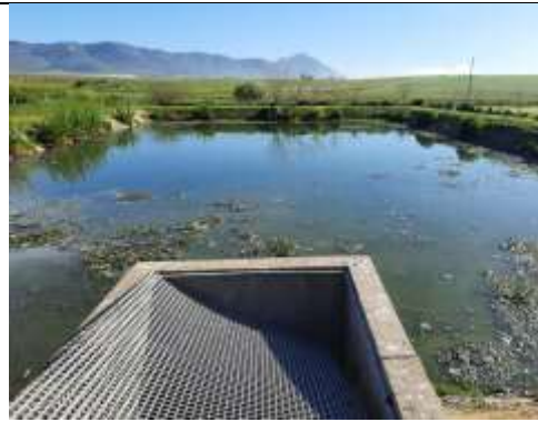
Dam receiving overflows is not in good condition. Sluice gates stolen and sludge build up noticed
