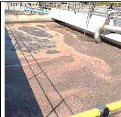
The plant uses fine bubble aeration in the bioreactors and in general a good distribution of air could be seen.
