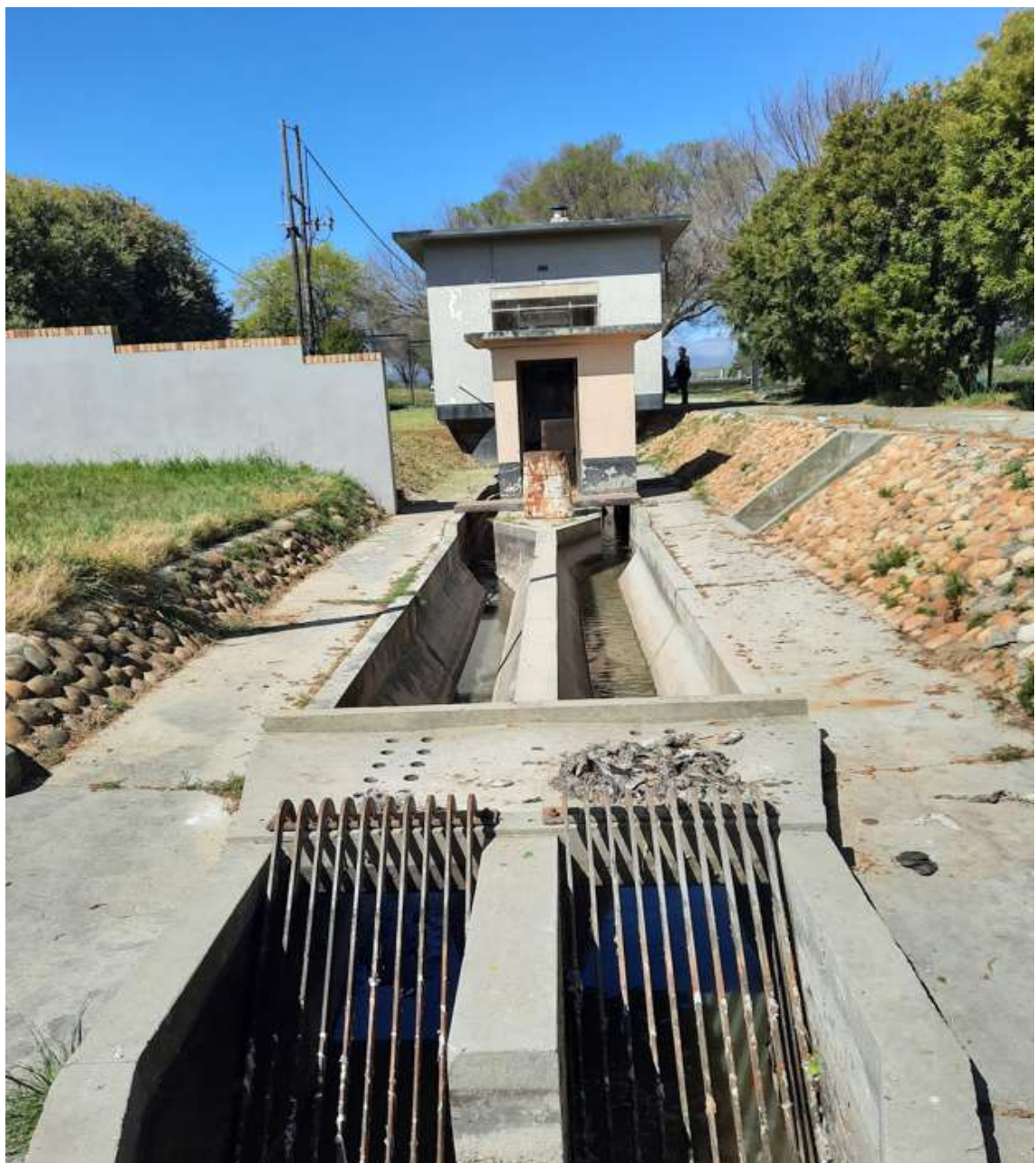
Witzenberg Municipality – a True Top Performer. A well-managed sewage transfer pump station on the outskirts of Ceres. All records of monitoring and management schedules are kept on site and clearly updated.
