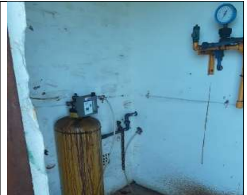
Chlorination room vandalised and stripped, not functional
