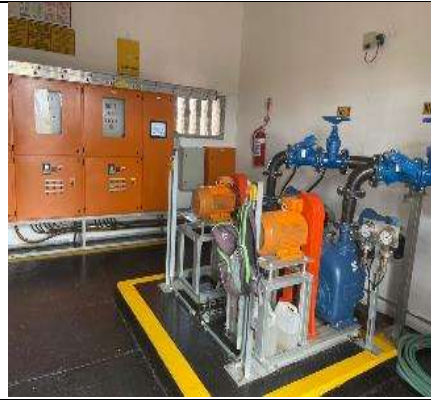
Network pump stations were in excellent condition
