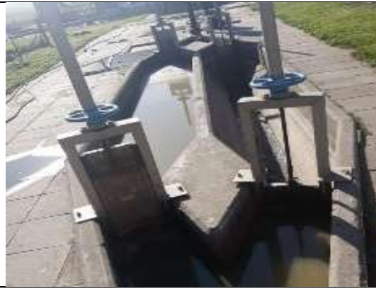
Flow meters and grit channels operational. Mechanical screen out for repairs, manual screen overloaded
