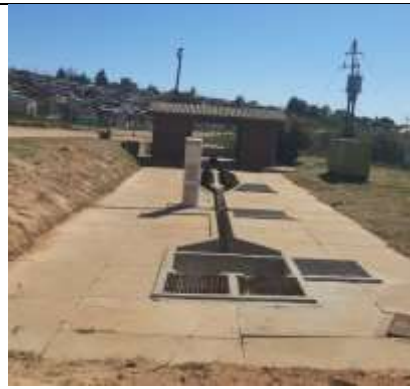
Inlet works equipment is in good condition
