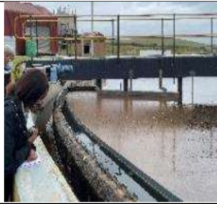
Some algae present on the settling tanks
