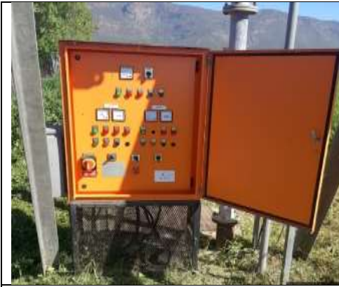
Electrical panels in good condition, all pumps functional without any downtime in 6 months
