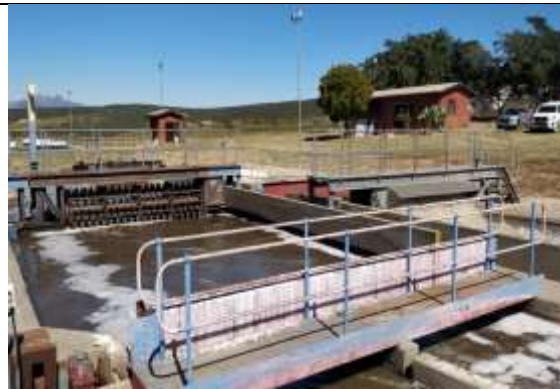
Activated sludge system is functional with RAS in place, but MLSS is not optimised
