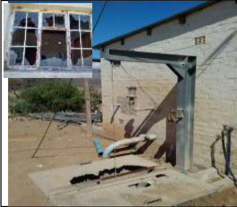
Pumpstation in poor condition, 1 pump functional, no signage
