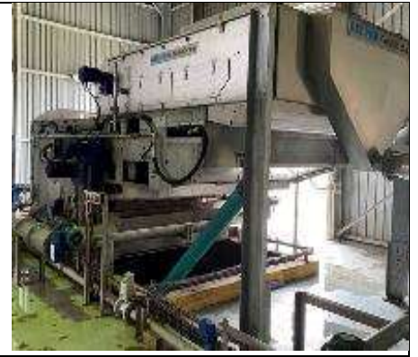
Sludge is dewatered with belt presses
