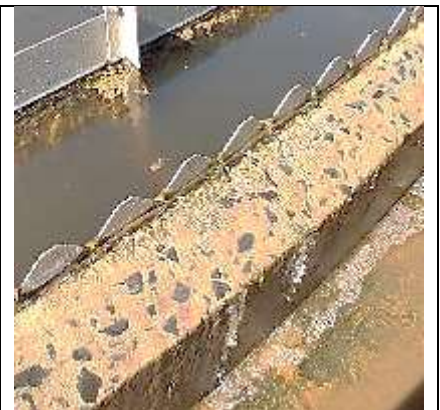
Minor corrosion on the concrete was seen in some areas and need to be addressed.
