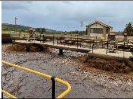
All mechanical equipment at the plant is in good working condition
