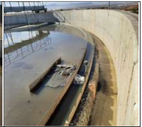
Scum withdrawal system not functional. Poor sludge settleability with pockets rising to surface
