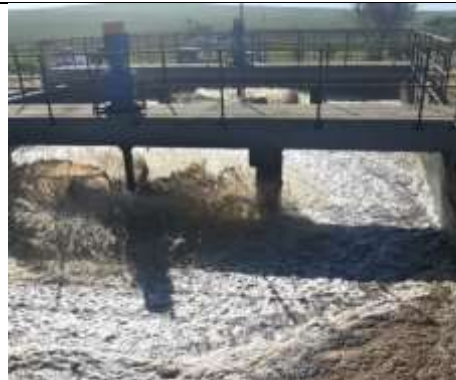
Aerators in new reactor functional, not in older module due to cable theft
