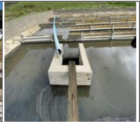
Final effluent channels are compromised by structural defects and Cl 2 system not functional
