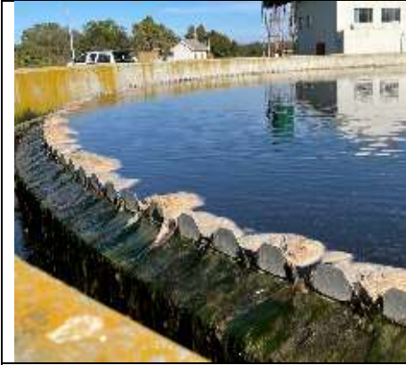
Good operational working of secondary settlers
