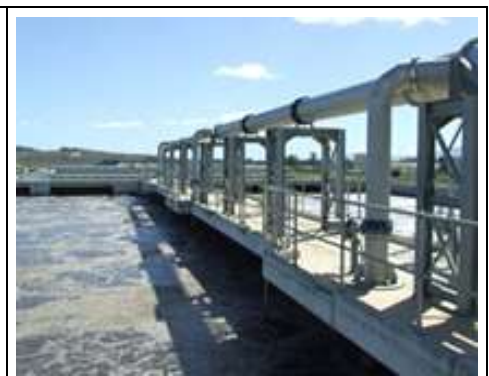
Activated sludge system is operational, with all operational controls in place – laboratory data used to optimise processes by knowledgeable staff.
