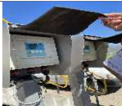
Flume with ultrasonic meter for inlet flow monitoring, verifying 44% of design capacity
