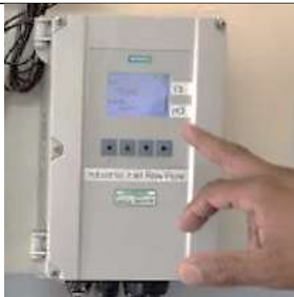
The plant is characterised by a number of flowmeters to gain more control over the operations of the works.
