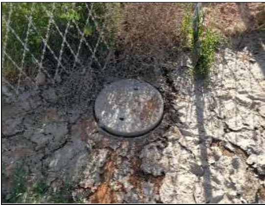
Spillages from manhole in sewer network, not cleaned
