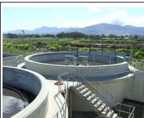
Infrastructure overall in good condition – electrical, mechanical and civil structures with functional SCADA control
