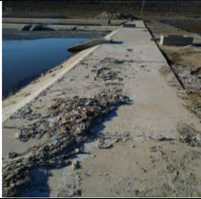
Debris is discharged on side of ponds, visually not appealing
