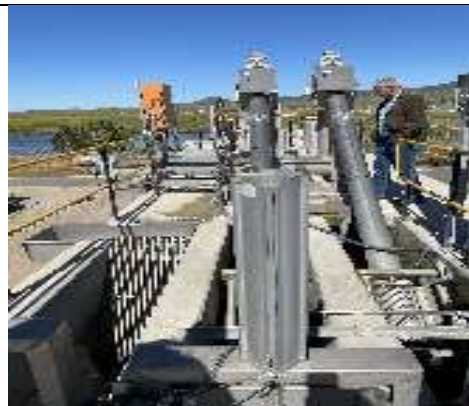
Mechanical screens functional and well maintained – good record keeping
