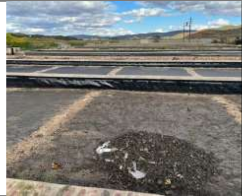
Drying beds were in clean and in good condition, with functional drains
