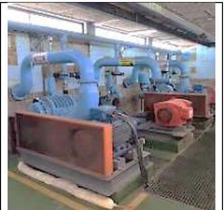
Effective operations and regular maintenance on all major equipment is seen at the plant
