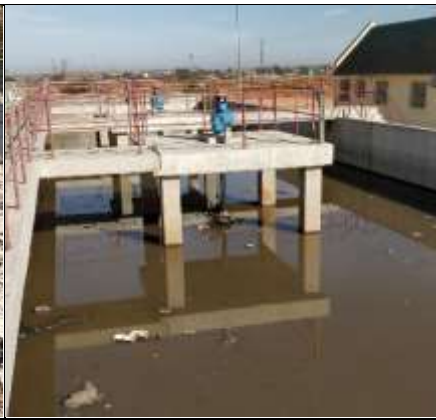
Three of 4 aerators are not functional, long lead times before equipment is repaired. No operational control
