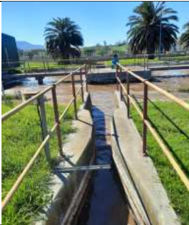
Grit removal functional, but terrain upkeeping needs attention
