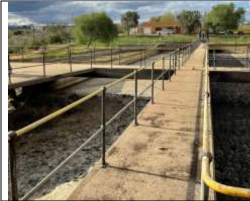
Excessive scum in the reactor affecting final effluent quality
