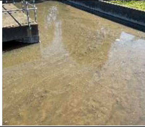
Several mechanical equipment at the plant is dysfunctional and compromise operations and compliance
