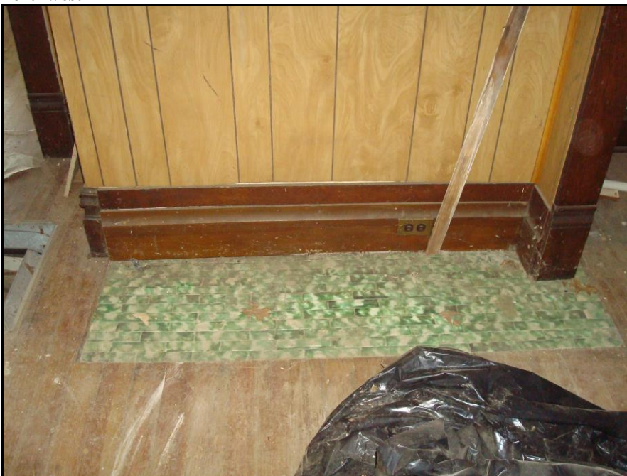
Photo 18. Tiled portion of floor in dining room, likely a closed up fireplace, first floor interior, facing north.
