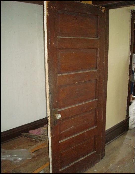
Photo 17. Original door between living and dining room, opening to hallway to the west, first floor interior, facing northwest
