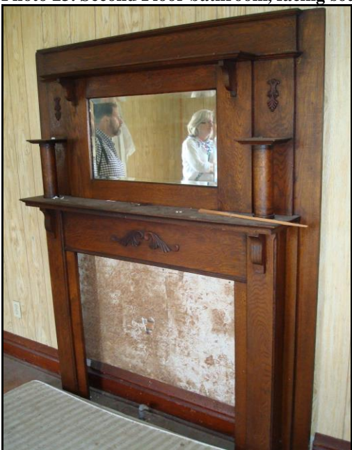
Photo 24. Fireplace mantel, second floor eastern front bedroom, facing north (possibly from first floor).
