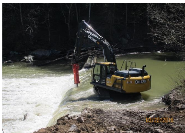
Figure 32. Removal of West Milford Dam, Harrison County, on the West Fork River in March 2016.
