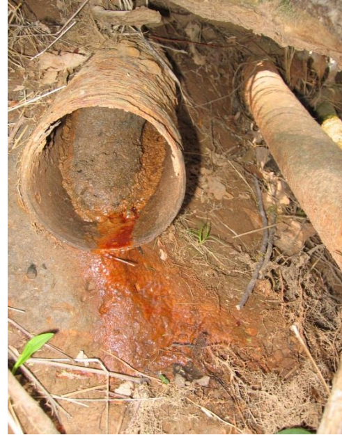
Figure 23. Leaky abandoned oil pipe in bank of Meathouse Fork of Middle Island Creek, Doddridge County.
