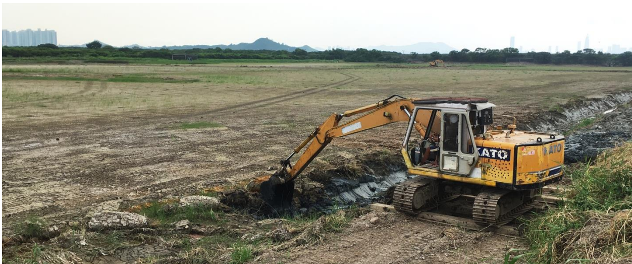
Desilting of gei wai channel, one of the major habitat management work in summer.
