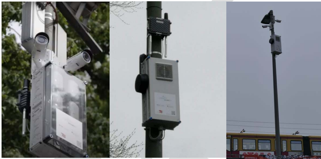
Figure 68: Three examples of the nine currently deployed eRSUs at the DE TS along Str. des 17. Juni in Berlin
