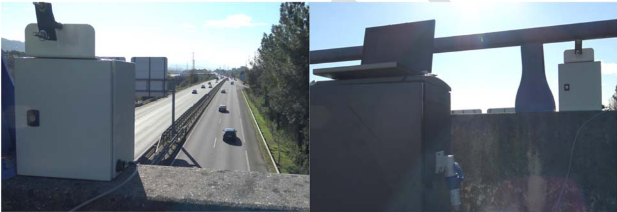
Figure 56: CTAG traffic radar installed in the AP9-A55 lane merge in Spain
