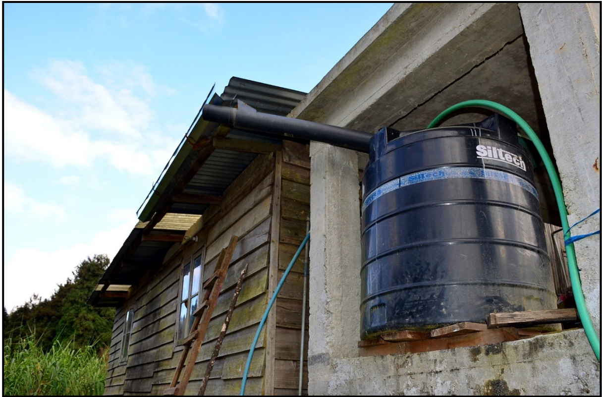
Figure 6. Roof top rainwater harvesting process at Chatakpur Village.
