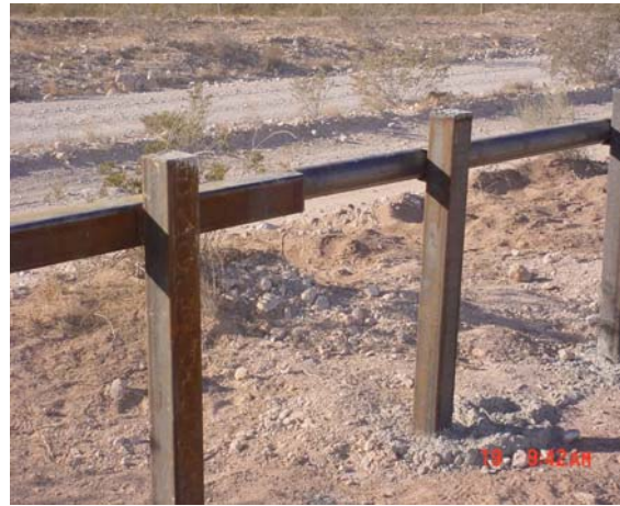
Photograph 2-1. Example of Post and Rail Vehicle Fence
