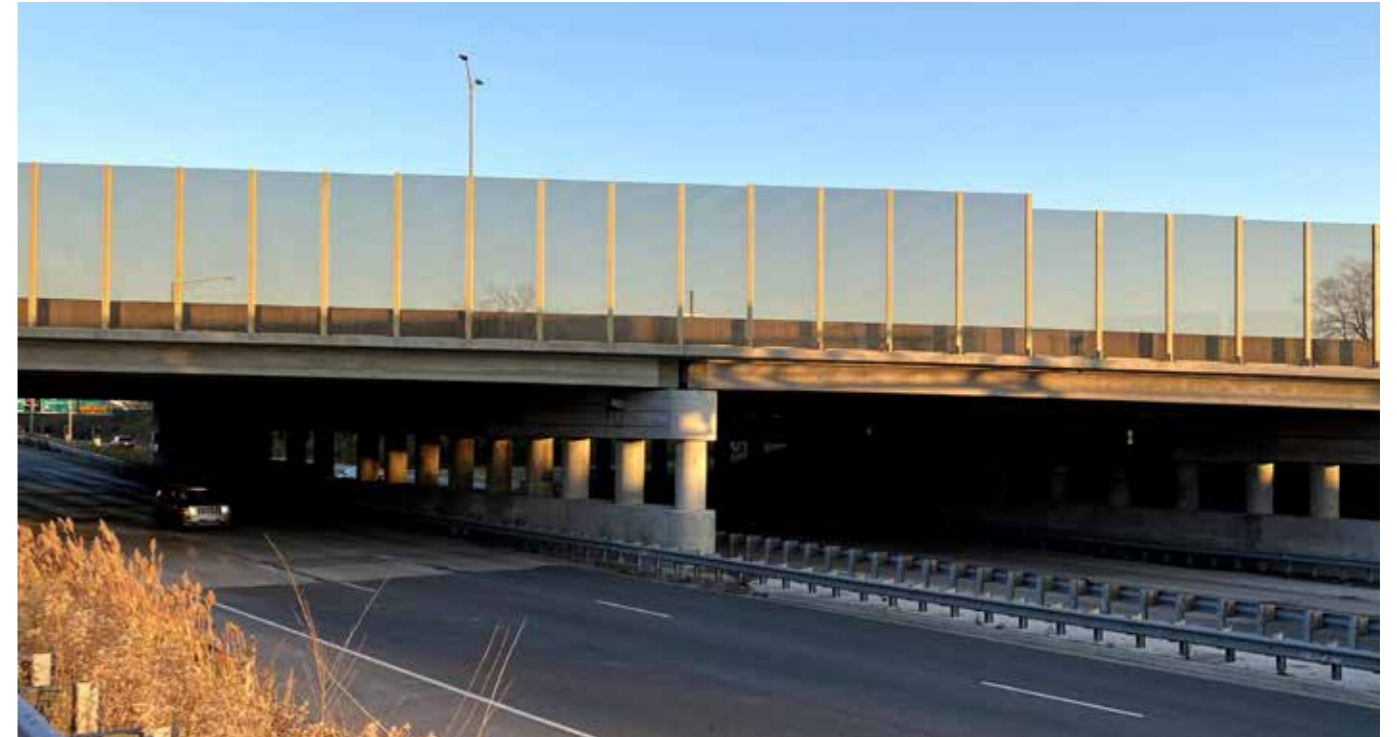
ACRYLITE® Soundstop GS CC Smoky Brown Structure Mounted System on I-88 over Roosevelt Road and IL-38 in Elmhurst, IL
