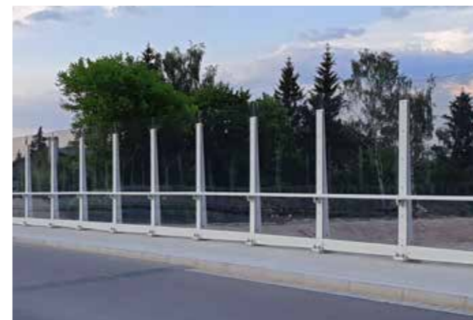
Noise barrier, Bridge Schwabach A6, Schwabach PLEXIGLAS® Soundstop GS CC
