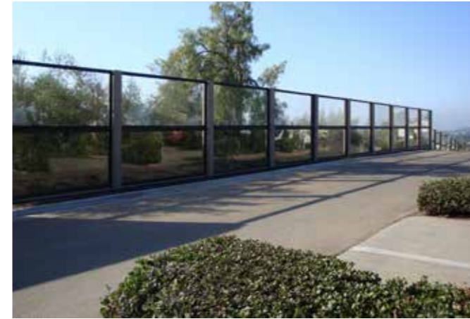
ACRYLITE® Soundstop Ready Fit System on Park Drive above the South Bay Freeway (CA-54) in Spring Valley, CA
