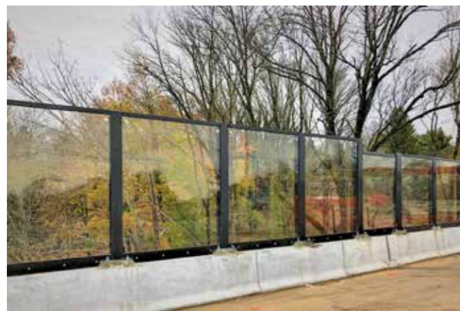
ACRYLITE® Soundstop GS CC Structure Mounted System on the Scudder Falls Bridge on I-295, Ewing Township, NJ
