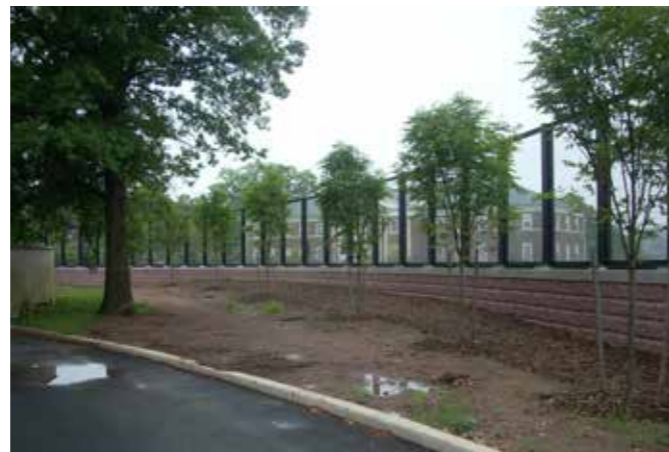
ACRYLITE® Soundstop Ready Fit System with black powder coated aluminum frames on Route 18 in New Brunswick, NJ
