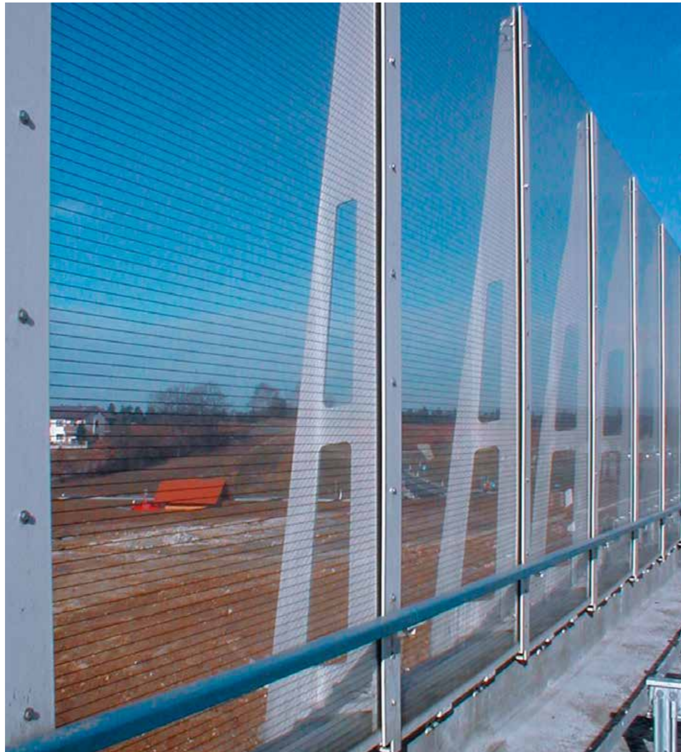
Noise barrier, Autobahn A9, Trockau PLEXIGLAS® Soundstop GS CC Fa. Markus Kaiser
