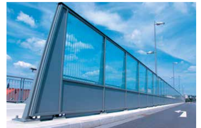
Noise barrier, Nibelungenbrücke, Regensburg Lower part made of PLEXIGLAS® Soundstop NT Fa. Markus Kaiser
