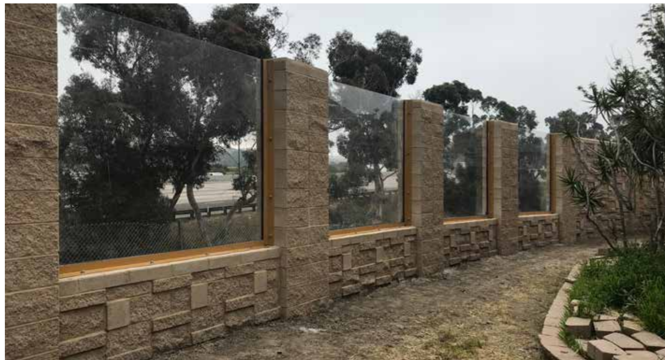
ACRYLITE® Soundstop CMU System with powder coated aluminum framing behind Nacion Ave off the I-805 Freeway in Chula Vista, CA
