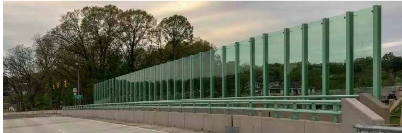
ACRYLITE® Soundstop GS CC Spring Green Structure Mounted System with green steel framing on the Peters Creek Bridge (NC-150) over US-158/US-421 in Winston-Salem, NC
