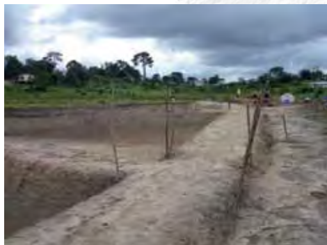
Photo E. Stakes put in while dikes are being built (Liberia) [© Y. Fermon].
