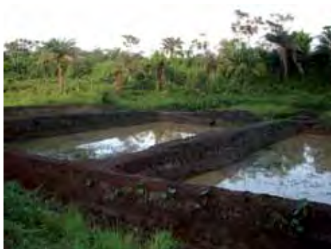
Photo B. Example of parallel rectangular ponds under construction (Liberia) [© Y. Fermon].
