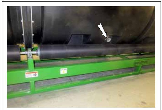
FIG. 17 TEMPERATURE GAUGE (TYPICAL)
