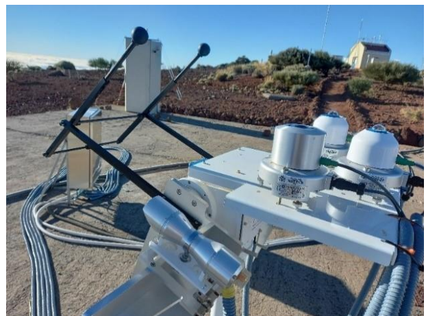
Figure 10.7. New instrumentation of the BSRN Izaña installed at IZO during 2022.
