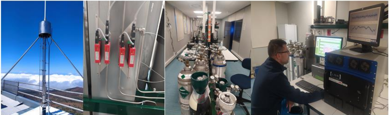
Figure 20.3. Ambient air/gas standard plumbing diagram of the Izaña-ICOS station. At the bottom, from left to right, photographs showing parts of the installation: sampling, flow meters, gas tanks and work station next to the instruments.
