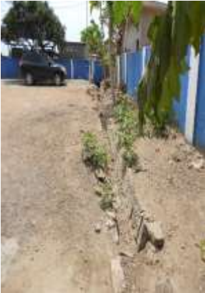
Damaged Drainage System
