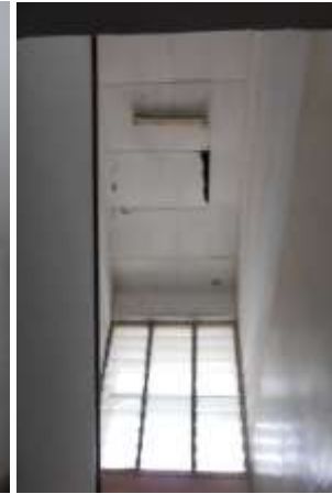
Damaged Overhead Ceiling
