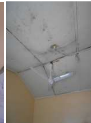
Damaged Interior Ceiling (2)
