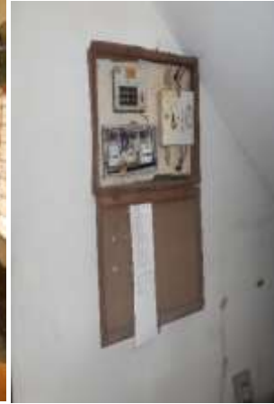
Uncovered Electricity Panel
