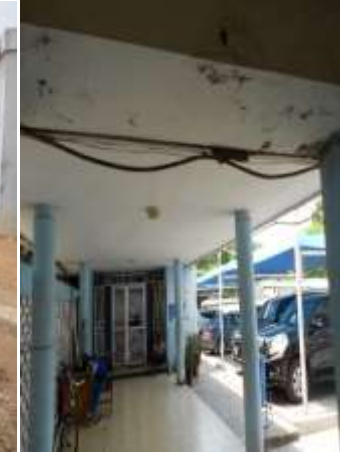
Hanging Electrical Cable
