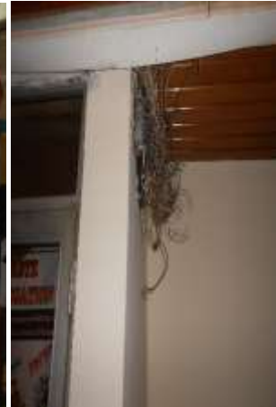
Exposed Electrical Wires
