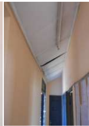
Damaged Interior Ceiling (1)
