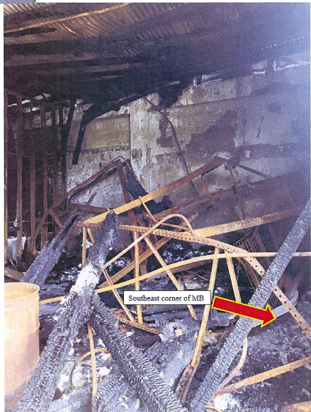
Figure 13: Photograph taken inside of MB on 31 July 2020 from south entrance depicting collapsed shelving and remaining metal barrel. (Tab Z-2)
