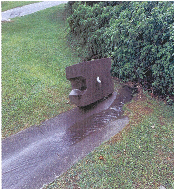
Figure 14: Photograph taken during stormwater outfall monitoring on 22 June 2020. (Tab W-23)
