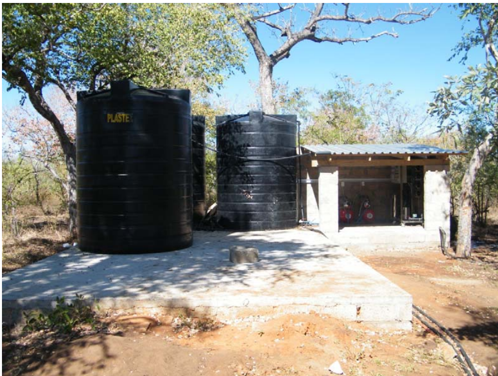
Water purification system at Buffalo Camp lodge
