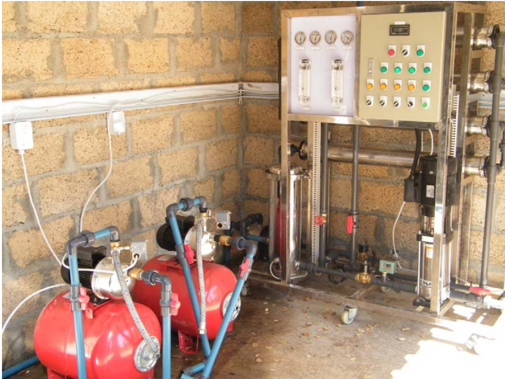
Control unit of the water purification system at Buffalo Camp
