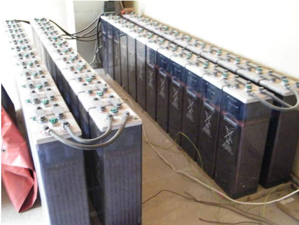
Solar power battery system at Buffalo Camp
