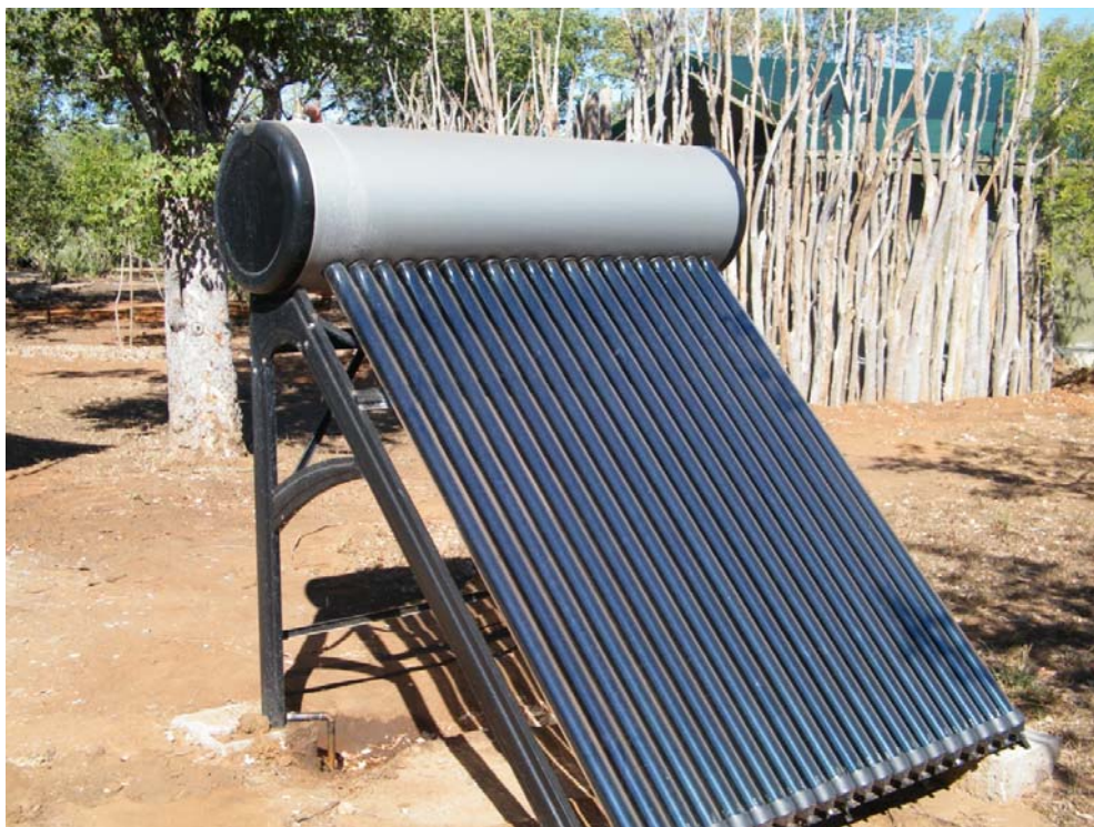
Solar power water heating at buffalo Camp lodge
