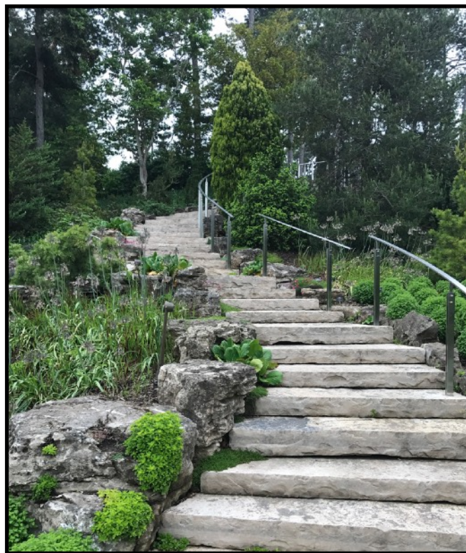
A main staircase had been degraded to the point of being unsafe. Image above is of staircase upon renovation completion. Image courtesy of Jon Peter.
