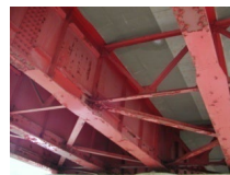
Bridge pier without Lumiflon® (16 years-old)
