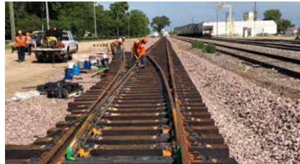
Switches from track 1 to track 2 are being installed in Dawson, Minnesota. Pending any weather delays, the track project will be completed in 2020.
