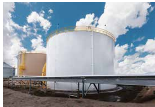
An expansion project underway at the AGP soybean oil refinery in Hastings, Nebraska, will greatly expand the amount of soybean oil storage.
