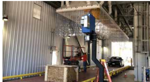
A crew works on interior upgrades to the truck loadout in Eagle Grove, Iowa, enabling soybean meal to be loaded at a much faster rate.
