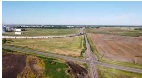
Dirt work began on a new rail project in Aberdeen, South Dakota, in mid-July. This is a view just east of the plant, looking west. At the bottom of the photo is the DMVW track being accessed.
