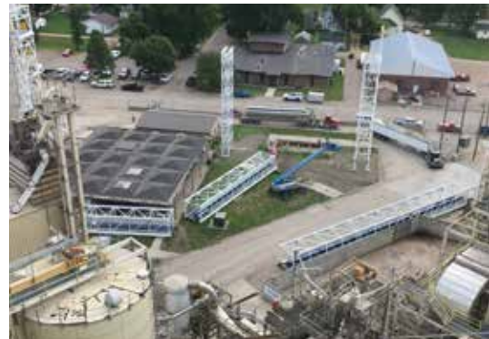
Some of the structural pieces, specifically bridges for lifts, have already been set for the first phase of the prep building upgrades in Dawson, Minnesota.
