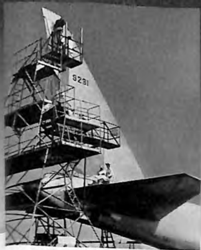
◀ Flight line work being done on B-52 tail. Tip is 48 feet above ground.
