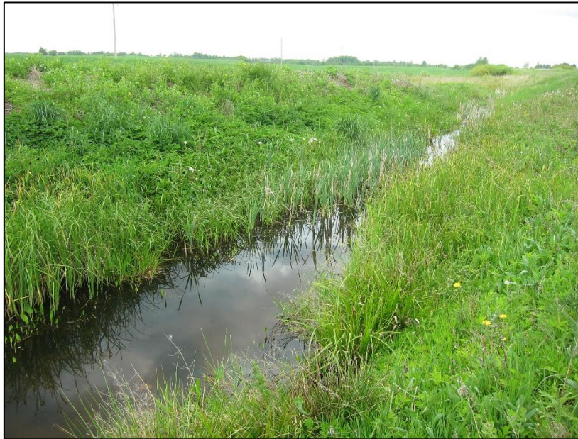
Figure 5.57: Overgrowing ditch extending along the road
