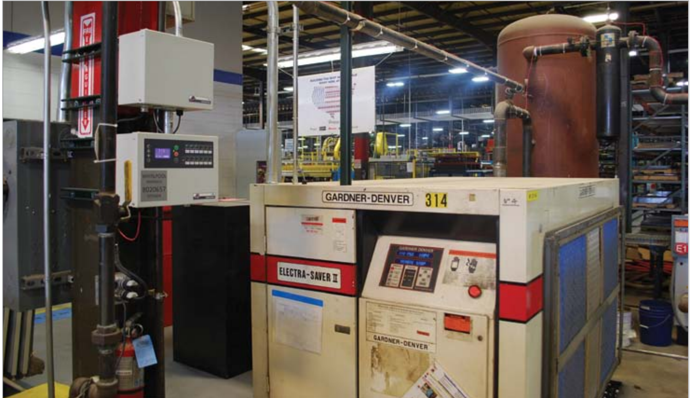
Measurements of compressed air pressure, flow and energy consumption were taken at the four separate air compressor installations.
