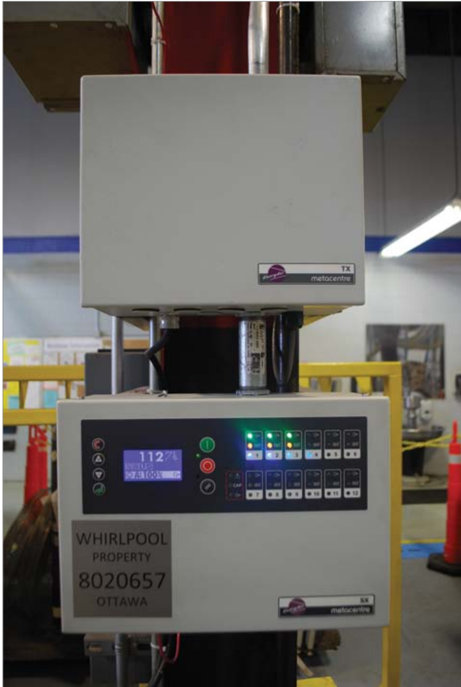
Metacentre TX, EnergAir’s dedicated host server provides remote access to Metacentre visualization screens allowing the performance of the compressed air system to be monitored and reviewed by employees at their desks.
