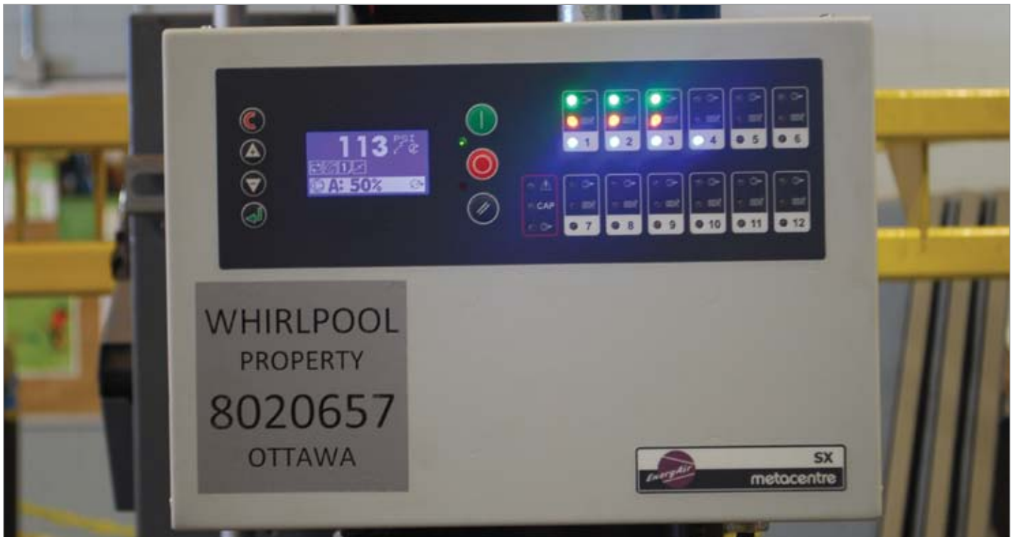
Before the installation of the Metacentre SX, multiple air compressors were running between shifts, during weekends and at other times when air demand was relatively low.
