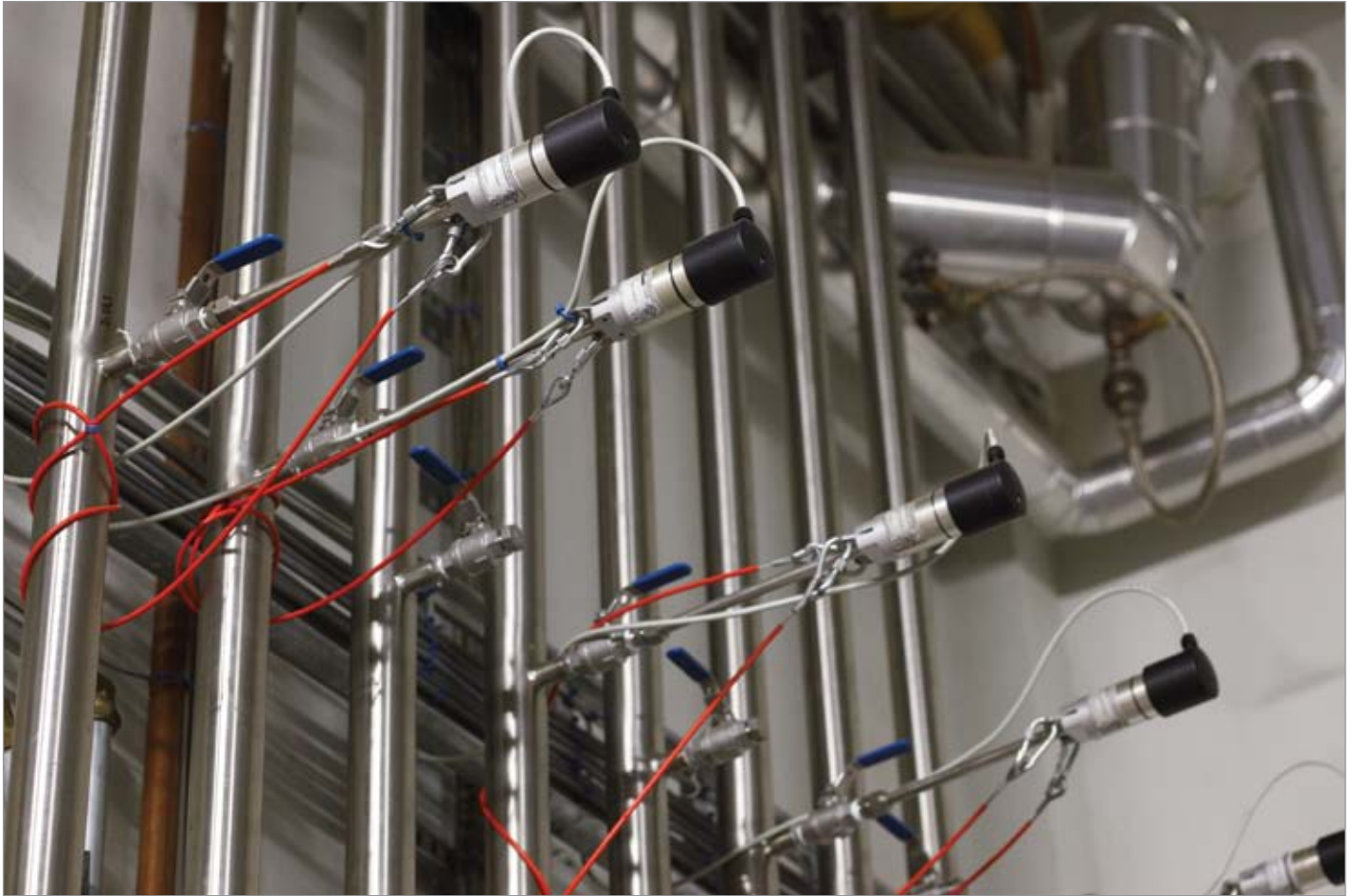
Measuring compressed air flow heading to different production areas
