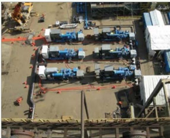
Aggreko supplied 150,000 scfm of oil-free compressed air to supplant a failed main air blower at a synthetic crude plant.
