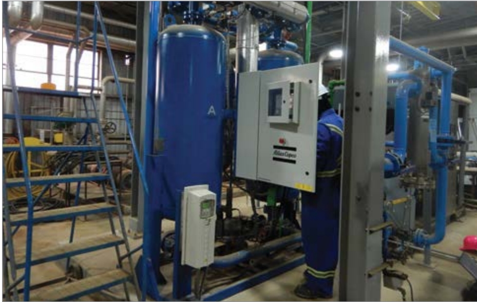
Figure 4: A new compressed air dryer has a closed cycle cooling circuit using no compressed air
