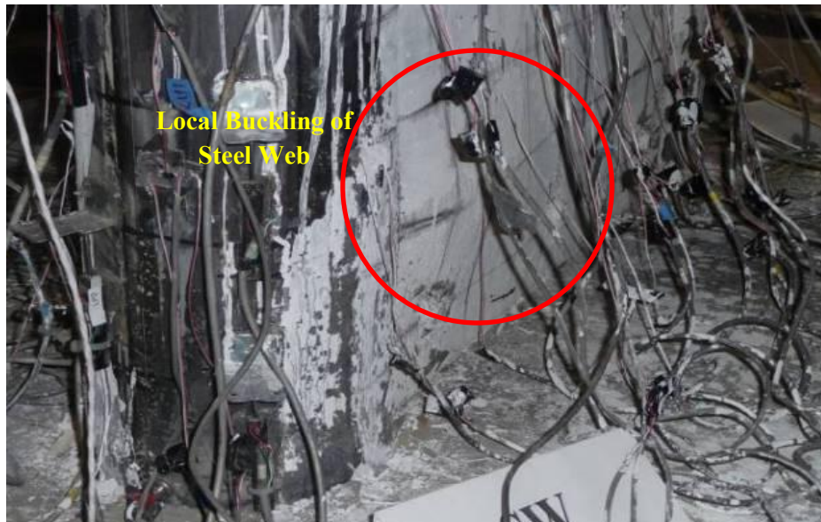
Figure 5-55 Local Buckling of Specimen CFSSP-B2 at 2.67% Drift
