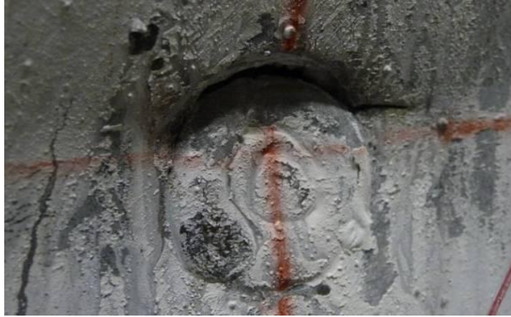
Figure 5-45 Fracture of Plug Welding of an Inner Tie Bar of Specimen CFSSP-B1 at 3.33% Drift
