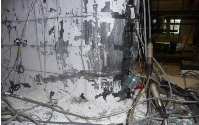
Figure 5-33 Propagation of Cracks in Specimen CFSSP-NB2 at 3.6% Drift
