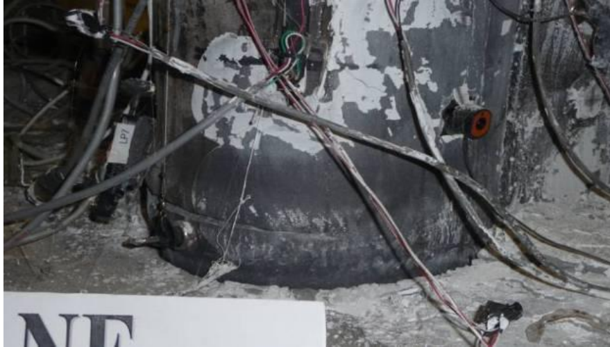
Figure 5-63 Fracture of the HSS Part of CFSSP-B2 at 4.67% Drift
