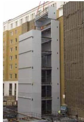
b) Corefast Walls used in Multi-story Buildings and Made of Bi-steel Panels
