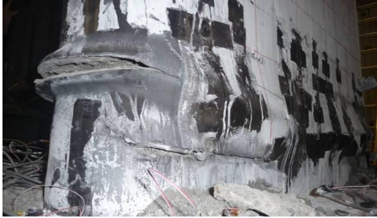
Figure 5-16 Fracture of the CFSSP-NB1 Specimen West Side at 3.6% Drift
