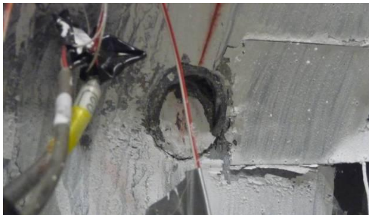
Figure 5-12 Plug Welding Fracture on the Full Diameter of the Tie Bar at 3% Drift
