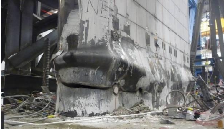
Figure 5-18 Propagation of Fracture of the CFSSP-NB1 for Specimen East Side at 3.6% Drift
