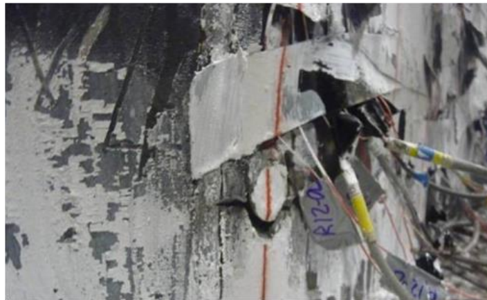
Figure 5-14 Propagation of Cracks on the West Side Tie Bar Circumference to CFSSP-NB1 Skin Plates at 3% Drift
