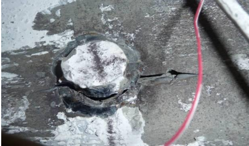
Figure 5-61 Propagation of Cracks at Outer Tie Bars in Specimen CFSSP-B2 at 4% Drift
