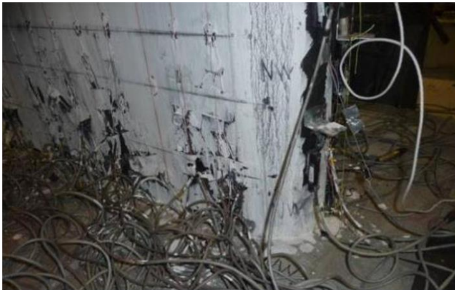
Figure 5-1 North West View for Specimen CFSSP-NB1 at 0.2% Drift.
