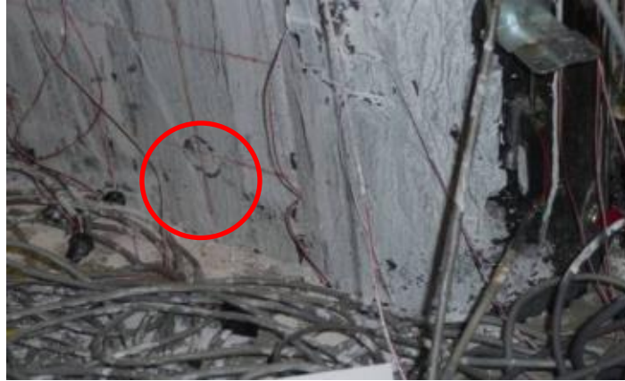
Figure 5-39 Full Diameter Cracks in the Tie Bars Plug Welding of Specimen CFSSP-B1 at 2% Drift
