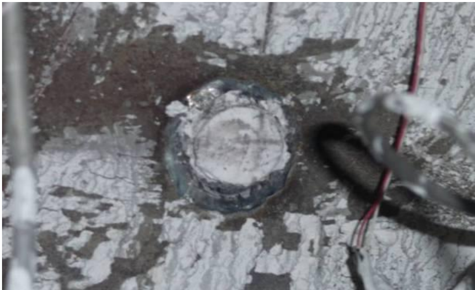
Figure 5-60 Intact Welding for Intermediate Tie Bar of Specimen CFSSP-B2 at 4% Drift
