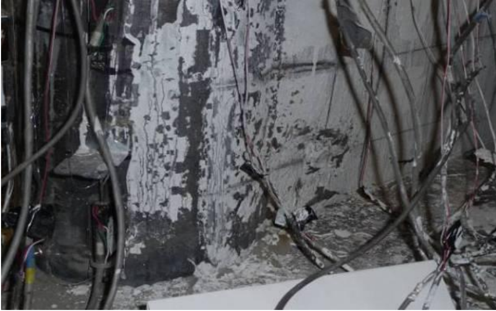
Figure 5-57 Local Buckling of HSS in Specimen CFSSP-B2 at 2.67% Drift
