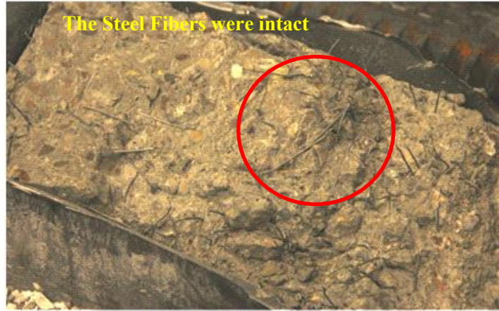
Figure 5-67 The Intact Steel Fiber Used in the Filled-in Concrete Mix
