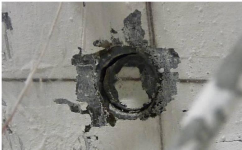
Figure 5-32 Failure of Plug Weld for Inner Tie Bars of Specimen CFSSP-NB2 at 3.0% Drift
