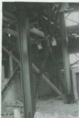
Fig.26 Buckling of Bracing Member
