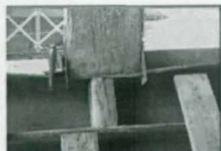
Fig. 1. Flange local bending in sill beam (courtesy of J. Lammers)
