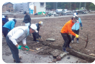
Clearing drains in a residential area (Ofunato, Iwate Prefecture). The mud is packed in sandbags.
