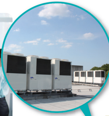
GHP installed on a building rooftop
