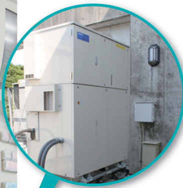
Commercial-use gas cogeneration system installed in a commercial facility
