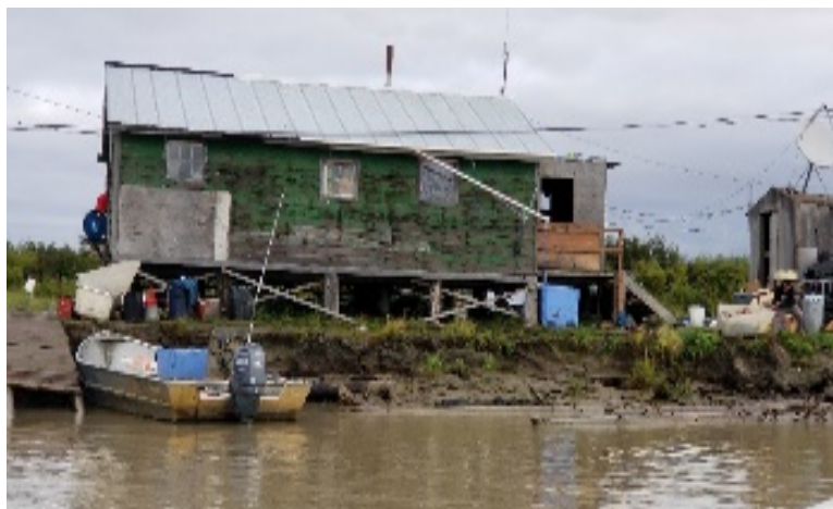
Figures 6-8: Three elders' homes immediately threatened by erosion that need to be relocated (Tanya Hunt, AIJ Personal Communications, August 2018).
