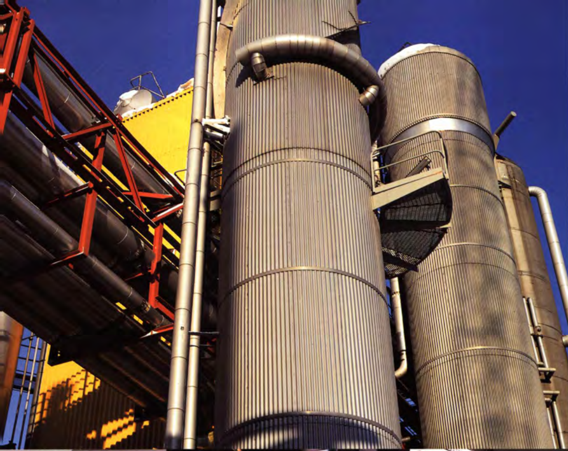
Akzo Nobel's hydrogen peroxide plant, Bohus, Sweden
