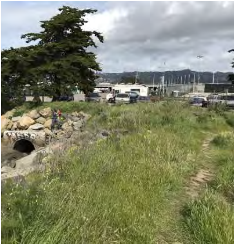
Photo 3: Photograph taken looking east toward outfall along Fleming Point (south of project boundary).
