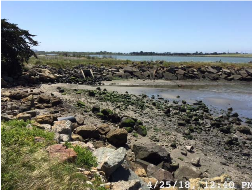
Photo 1. Looking South toward 60-inch Culvert Outfall at the end of Gilman Street during Low Tide
