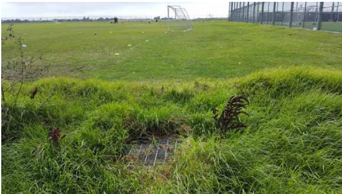
Photo 4. Drainage Grate at Northern End of Depression 1, facing west
