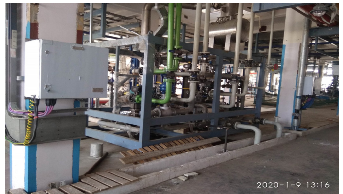
Figure 2: Field junction boxes are located near the sensors and actuators wired to them.
