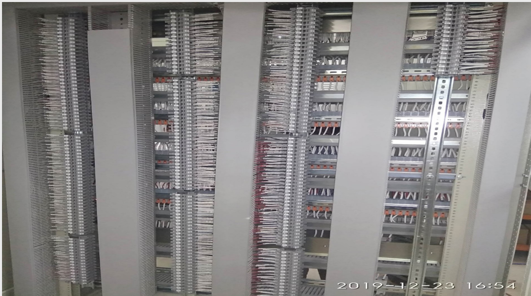
Figure 4: The marshalling cabinet is where the field wiring and system cabinet wiring are interconnected.
