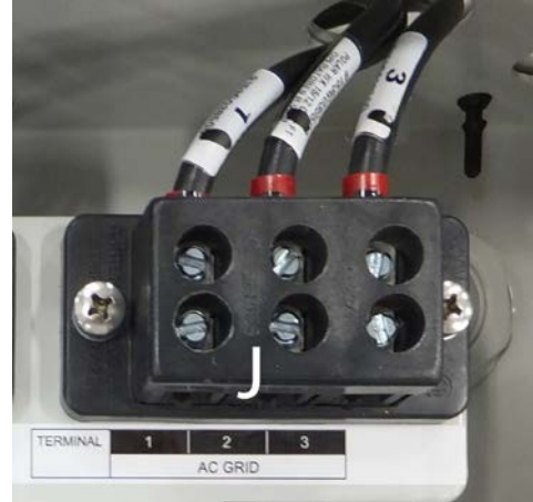
Figure 3-18: Bottom switch AC grid terminal
