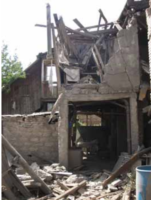
A house in Tskhinvali , South Ossetia, destroyed by a GRAD missile. ©Amnesty International
