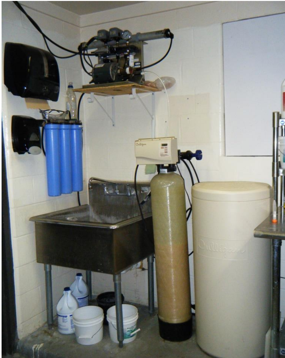
Figure 1. Sink and water treatment area for each room
