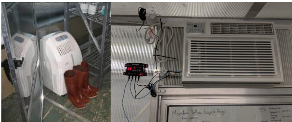
Figure 3. Left: The portable heating/air condition unit and dedicated footwear placed in each room. Right: Combined heating/cooling window units added above the door frame to provide colder temperatures. A CoolBot controller (seen to the left of the unit) has been added to the unit to achieve temperatures as low as 38F.
