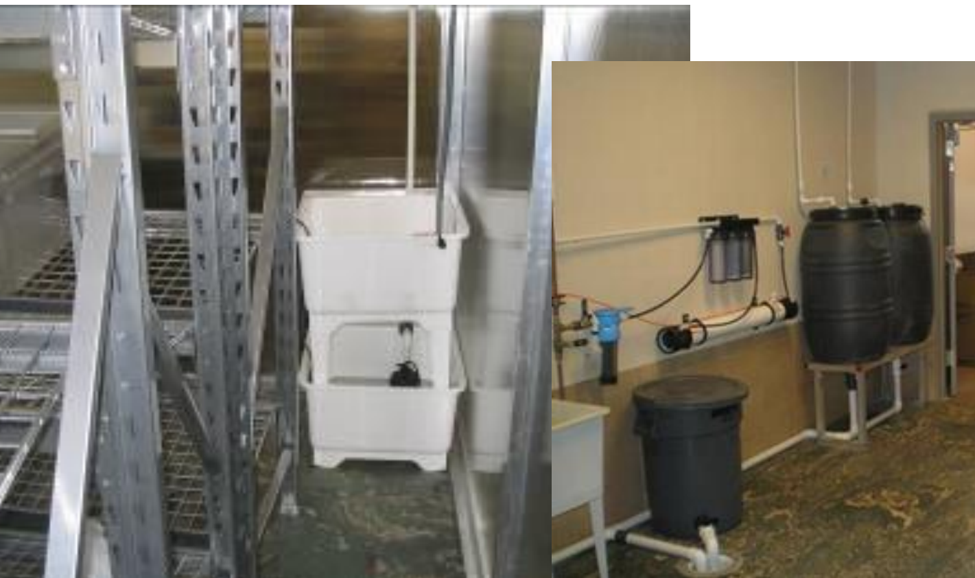
Figure 8: Left: Stacked room wastewater collection tubs with sump pump below to pump water to the central treatment station. Right: The two black barrels serve as the central treatment station for the entire area allowing for wastewater disinfection before release into the municipal wastewater system through floor drain. Note: All drain pipes are thoroughly-directed into the tubs/barrels/drains to minimize splashing of potentially diseased or chemically contaminated wastewater.
