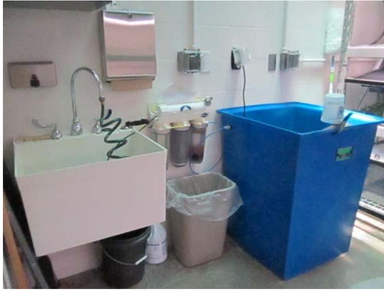
Figure 4. Service area within each quarantine room includes a cabinet, sink, hose, and water filtration/storage vat.
