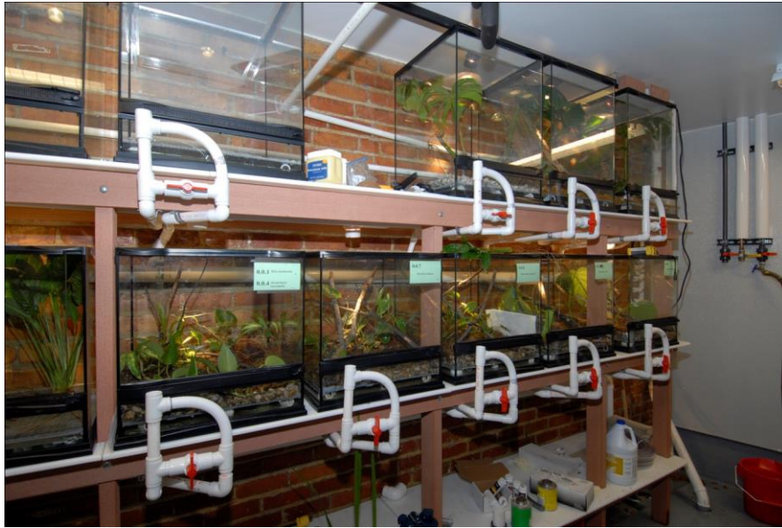
Figure 3. Each tank had its own standpipe overflow created out of “T” and flexible PVC, serviced by a quick-drain valve. All these drains flowed into a two-inch common drain pipe created by drilling a hole in the pipe and loosely fitting the 3/4-inch drain into the pipe. This prevented siphoning between cages.
