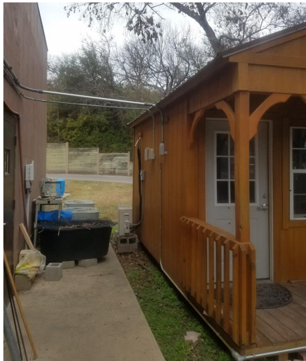
Figure 1. Overhead lines from nearby building provide electricity for the shed.
