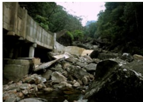
Figure 12. Hydroelectric power plant (note: concrete wall built across the stream and concrete particles dump in to the stream). Photo: Suranjan Karunaratna.
