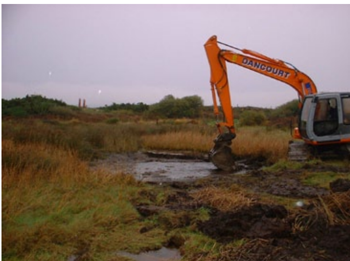
Figure 2. Excavating a new pool at Glenbeigh marsh in 2006 as part of a Biodiversity Fund project. Photo: William Shaw.
