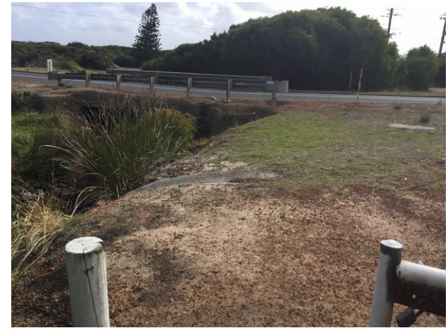
Bare and eroding banks needing revegetation
